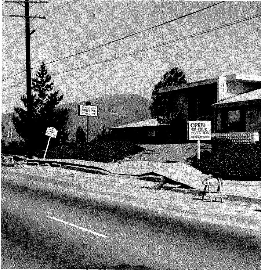
Figure I-5: Surface Fault Break. Area beyond curb was raised about 3 feet relative to the street. Unoccupied nursing home was damaged but did not collapse. (Los Angeles City Department of Building and Safety photo)
