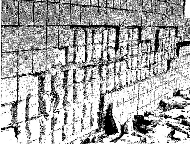
Figure 7 Investigations are needed to improve bonding the face shells of concrete block to the grout core. Note the horizontal pour joint in the grout cores.
