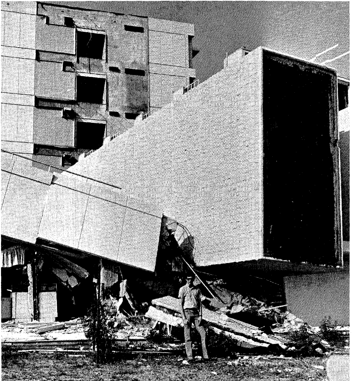
Figure A. Damage to Olive View Hospital building during the 9 February 1971 San Fernando earthquake. The earthquake design criteria for this building were not proper for such strong ground shaking.
