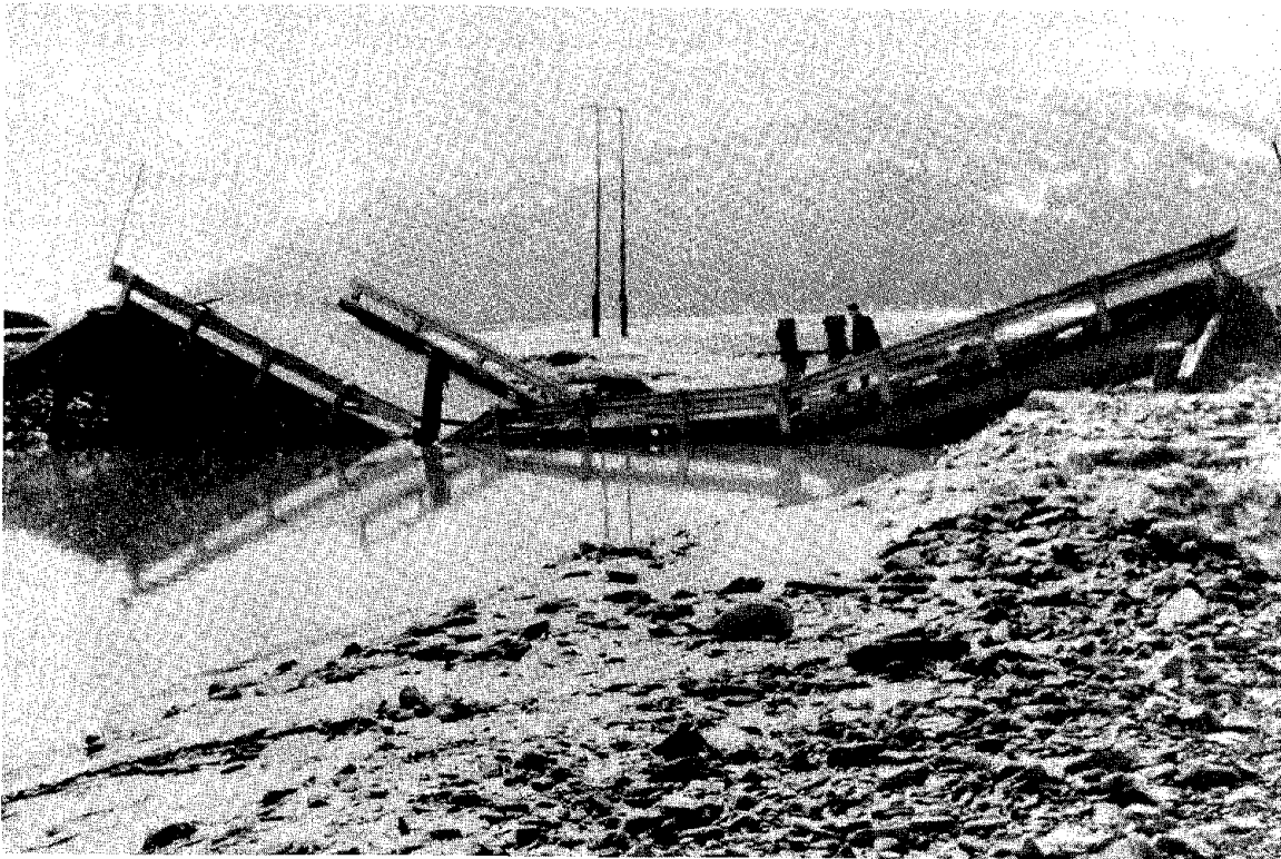
Collapse of a bridge during the Alaska Earthquake of 27 March 1964. During the earthquake the soft soil lurched and slid, pushing the bridge off its supports.
