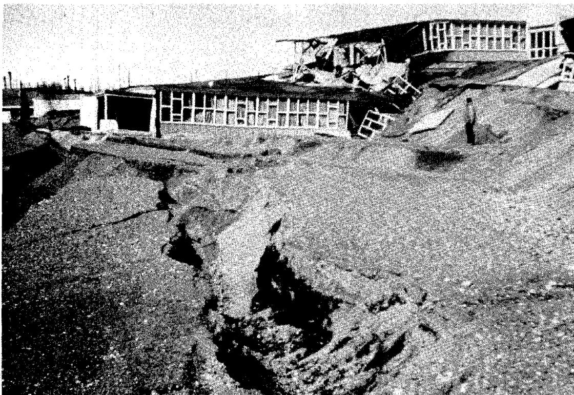
Collapse of school building as a result of the 1964 Alaska Earthquake.
