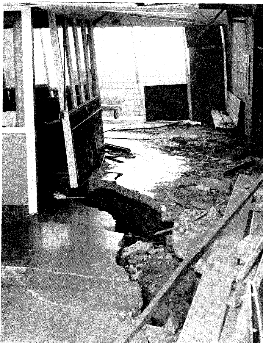
Structural damage to the juvenile hall resulting from ground cracking associated with land sliding during the February 9, 1971, San Fernando Earthquake.
