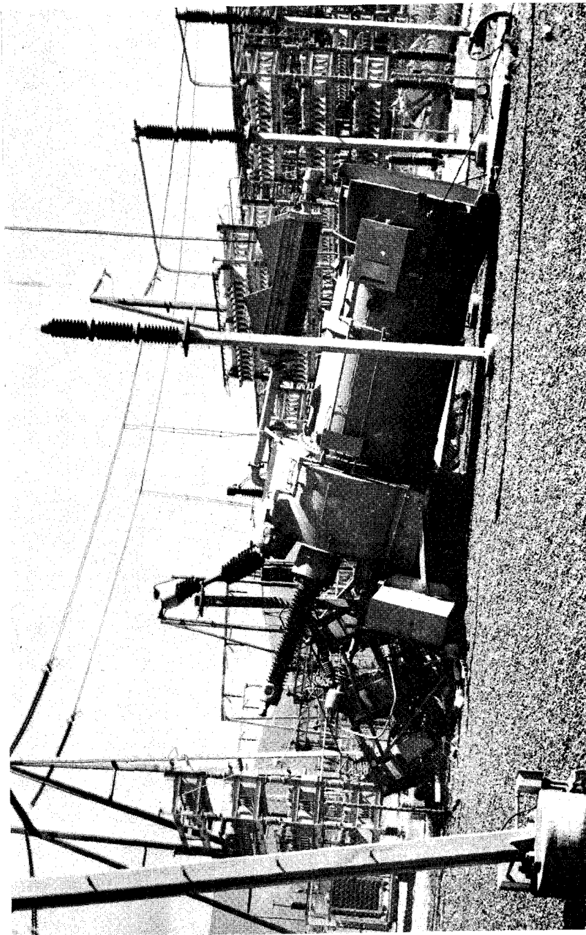
Overturned transformer at a major electrical converter station as a result of the San Fernando Earthquake, February 9, 1971, magnitude 6.6.
