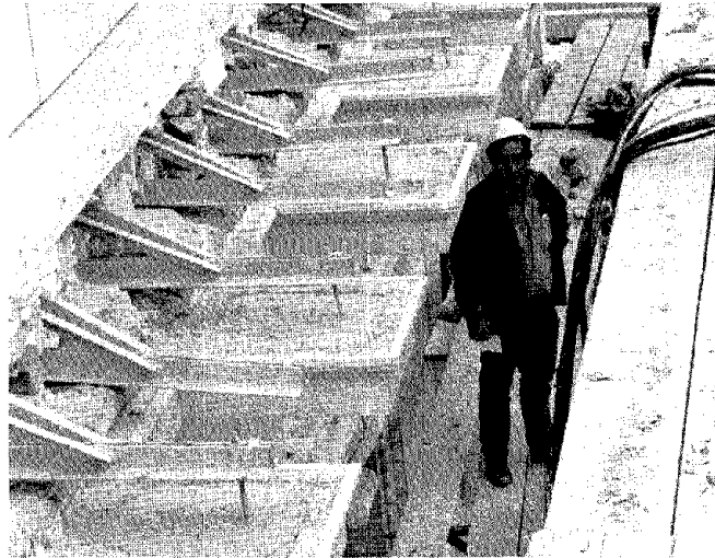
Figure 17 — Steel cornice anchors. Following setting of remaining terra cotta cornice elements, entire section will be filled with epoxy-ceramic foam for additional stability and protection from corrosion.
