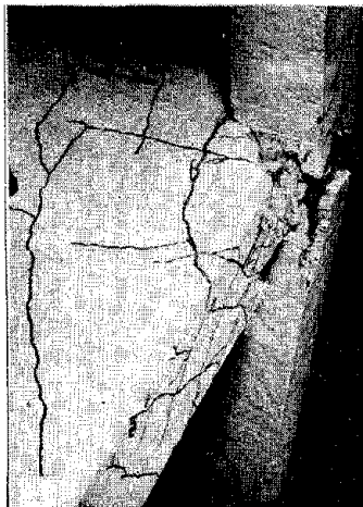
Fig. 25 Corner Joint of Model Reinforced Concrete Building Showing Diagonal Tension Cracks in Transverse Beam [55]
