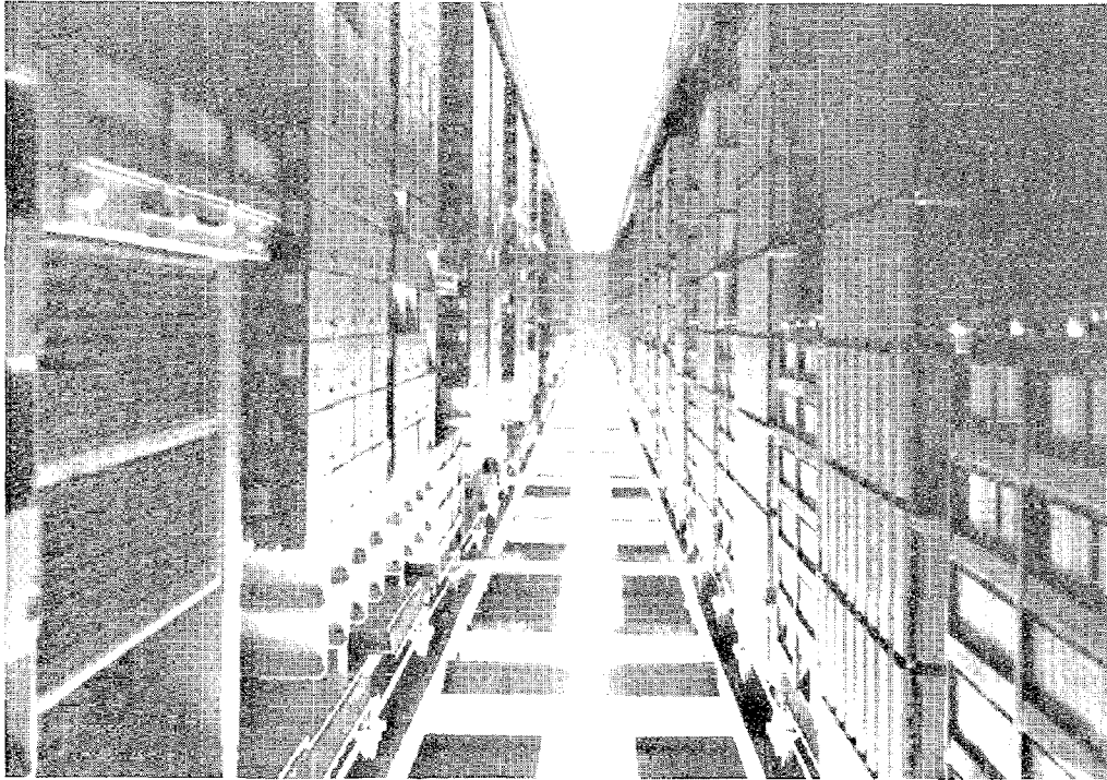
Figure 7. Typical 7-ft Electronic Equipment
