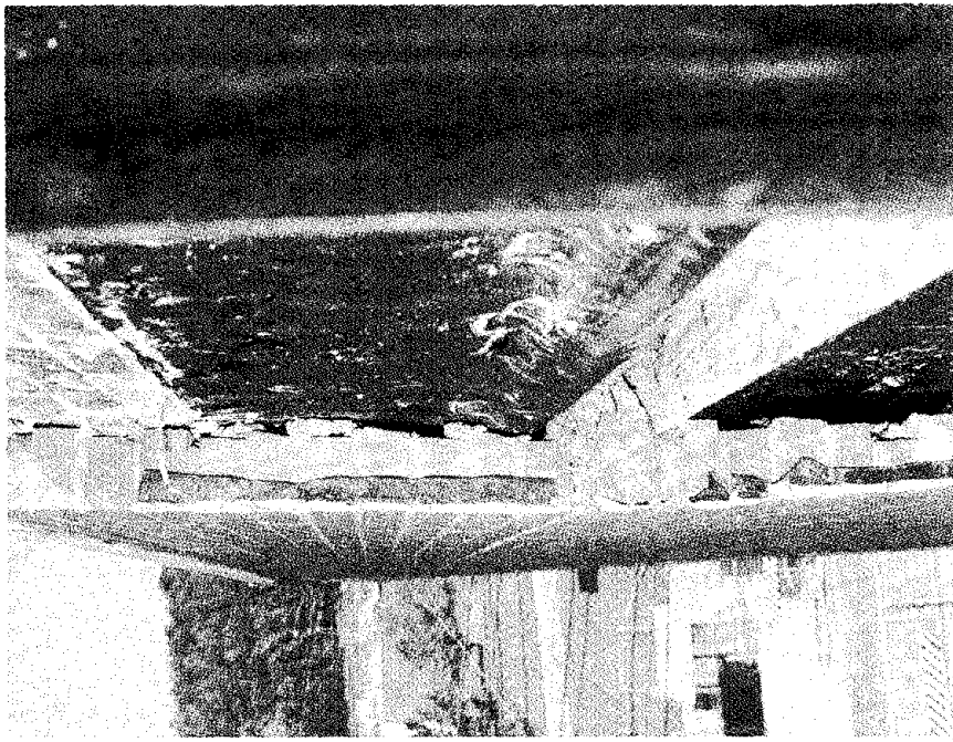
(a) WALL BULGE
