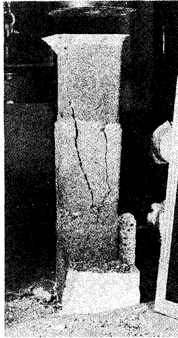
Fig. 4. Grout Core Splitting
