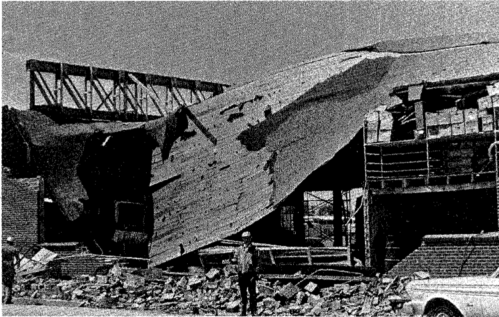
Figure 3 Marginally-Engineered Buildings Such as This Loadbearing Masonry Structure in Lubbock, Texas (USA) Perform Poorly in Extreme Winds.
