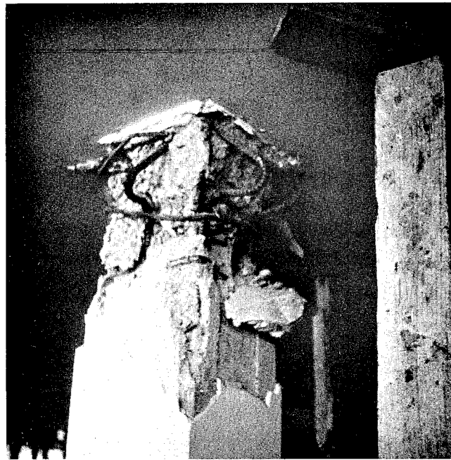
Figure 31 Axial compression failure of third-floor column of business house, Córdoba.
