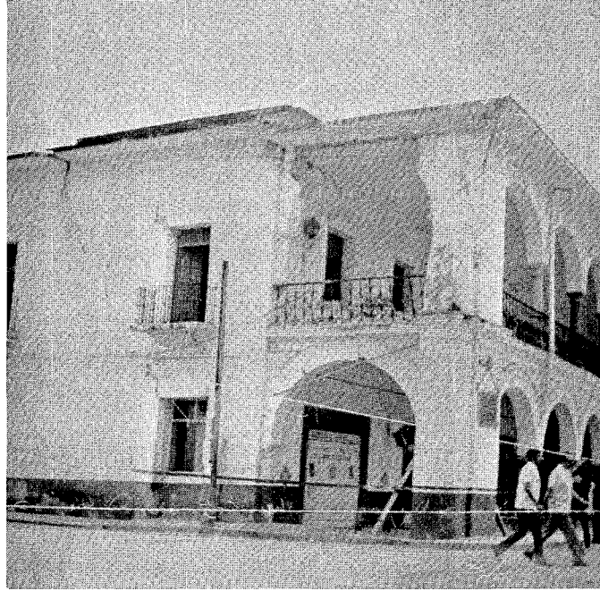
Figure 38 Damage to exterior corner of the Hotel Zevallos, Córdoba.
