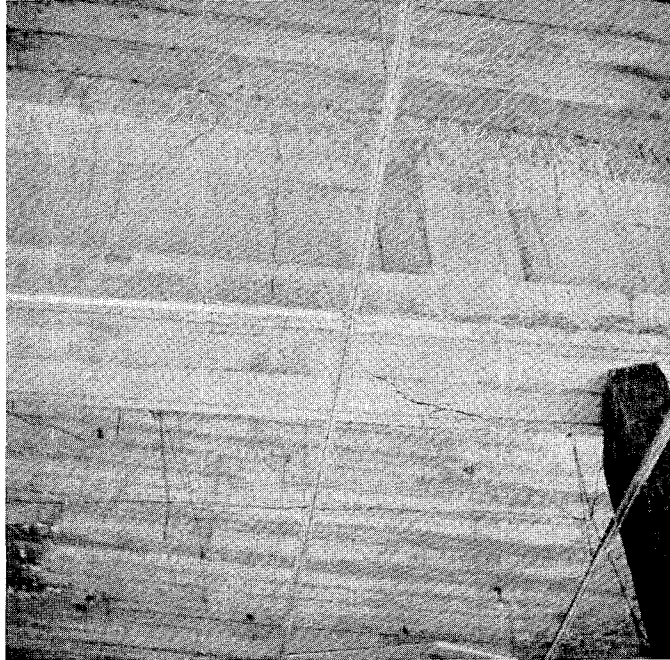
Figure 26 Flexural cracking at midspan of roof beam, VW Garage Showroom, Orizaba.
