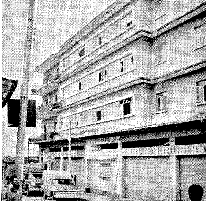
Figure 42 Apartment building, Córdoba. There was extensive internal structural damage to this building.
