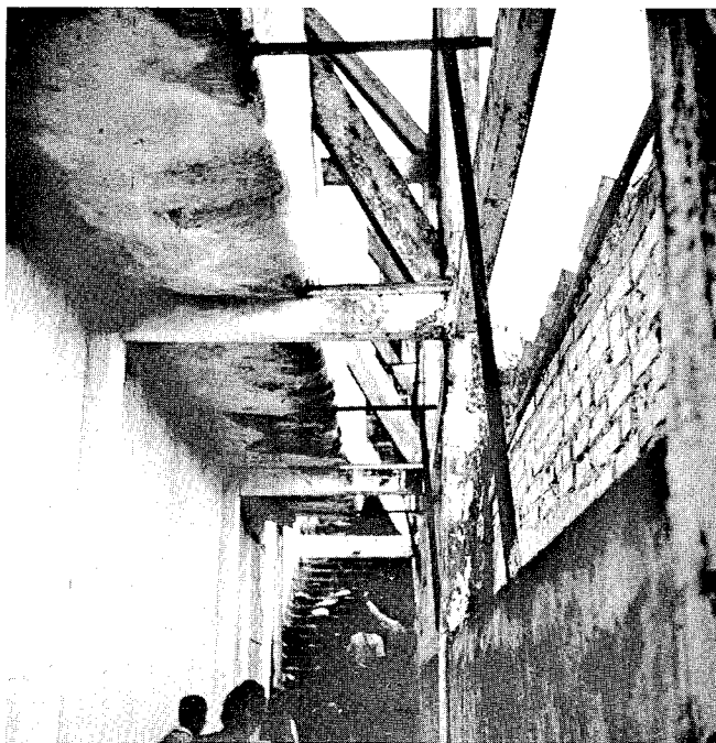
Figure 29 Damage to buttress frame, Cinema Real, Orizaba.
