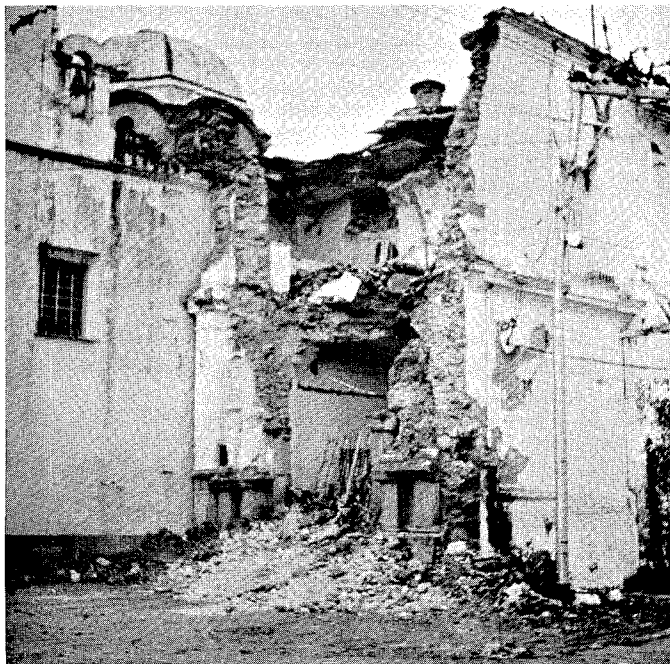
Figure 27 Damage to a church-hospital in Orizaba.
