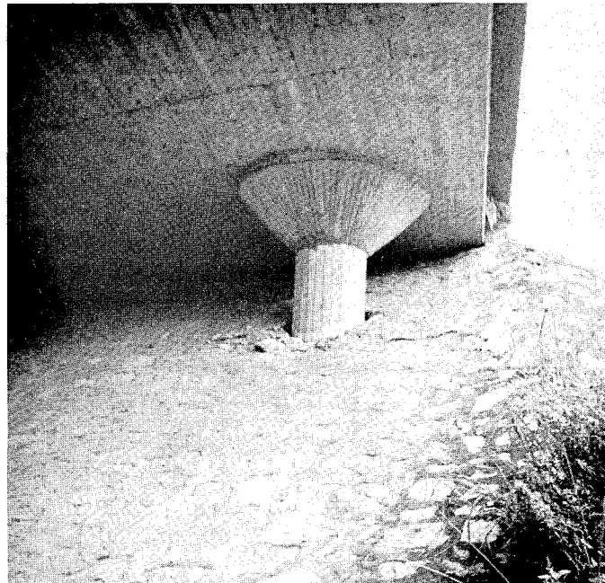
Figure 47 Settlement of embankment around bridge pier, Córdoba.
