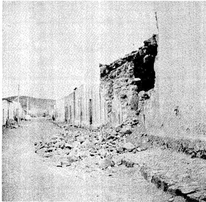
Figure 48 Typical view of damage to houses in Serdán.
