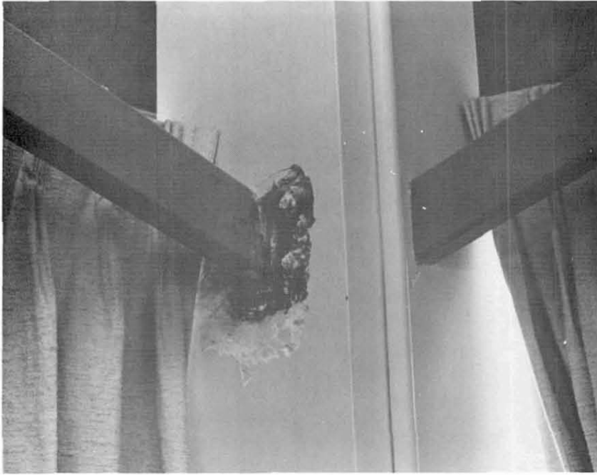
Figure 7.62 Close up of damaged joint shown in Fig. 7.61
