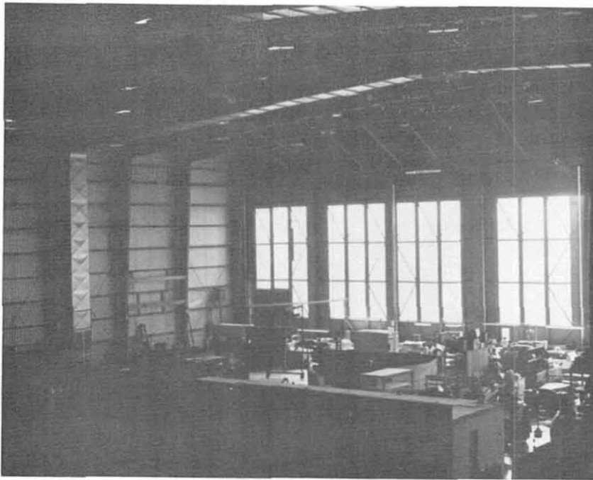
Figure 7.66 Interior of large hangar at facilities of Aero Spacelines, Inc., showing large sliding doors and damaged steel bracing which angles up to the roof from the rail at top of doors
