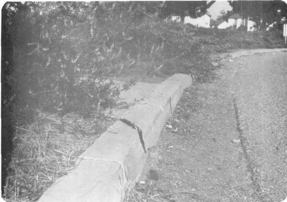
Fig. 9.10 Close up of curb push out shown in Fig. 9.9. (View from south.)
