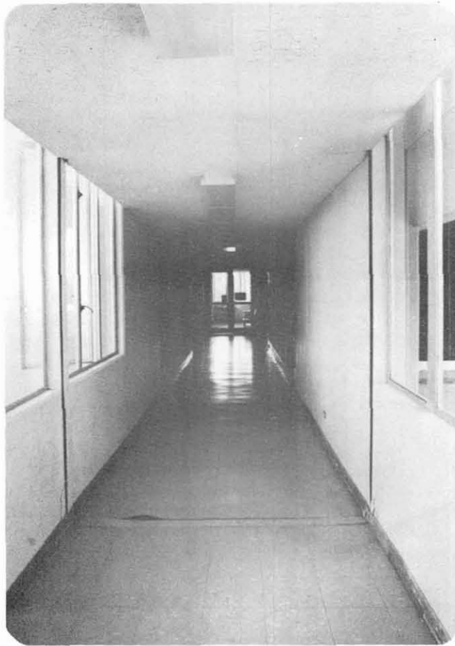
Fig. 11.1 Damage to seismic joint in South Hall, UCSB.
