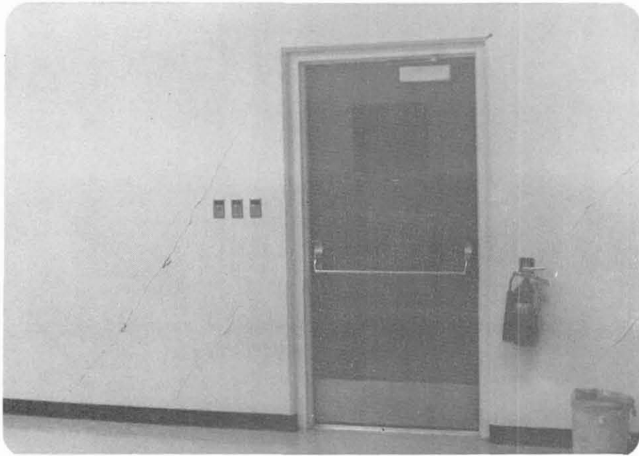
Fig. 7.29 Diagonal cracks in east-west shear wall in first story of Engineering Building, UCSB.
