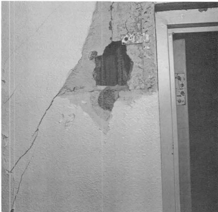
Fig. 7.23 Another example of ungrouted reinforcing steel, shear wall in Anacapa Residence Hall.
