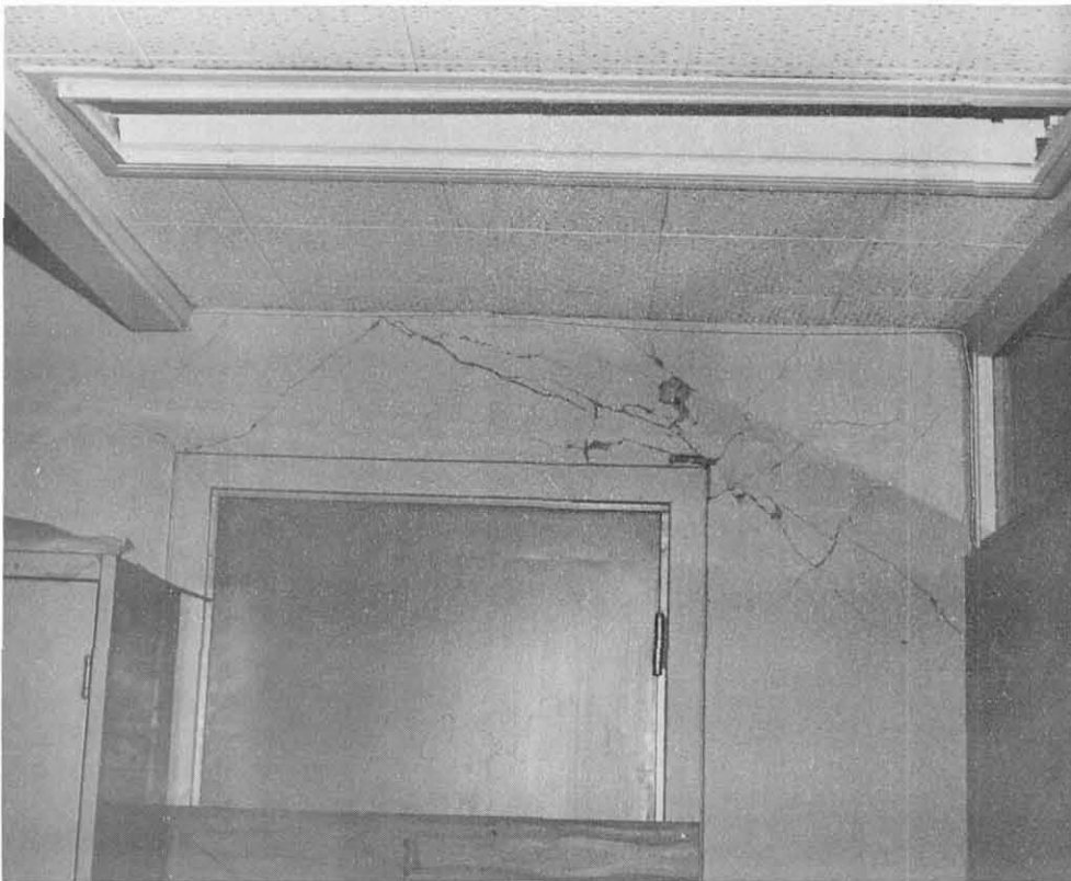
Fig. 7.43 Cracks in reverse side of shear wall shown in Fig. 7.42.
