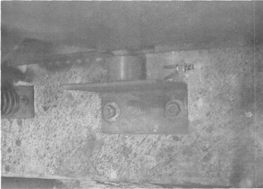
Fig. 8.21 Close up of commercially available seismic restraint on fan (Fig. 8.20).
