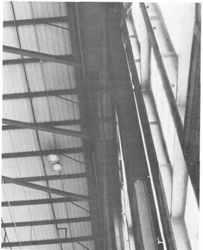
Figure 7.67 Close up from directly under damaged steel bracing of sliding doors shown in Fig. 7.66. Note separation of rail and bracing in center of picture
