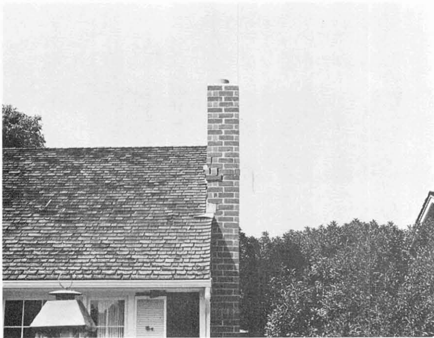
Fig. 7.52 Damage to chimney on modern residence in Isla Vista.
