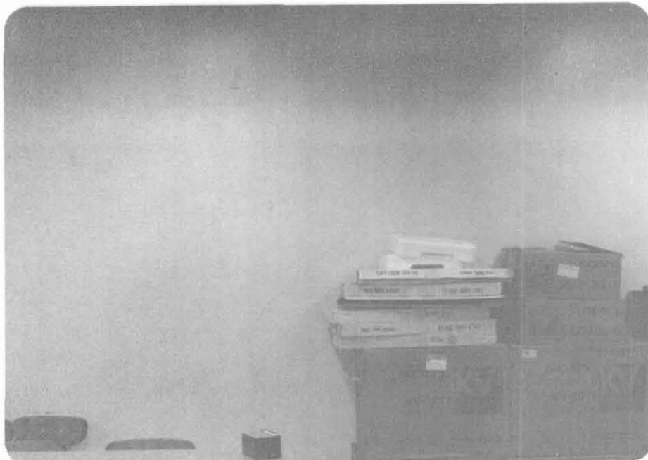
Fig. 7.30 Cracks in another portion of the north-south shear wall in the first story of Engineering Building, UCSB.
