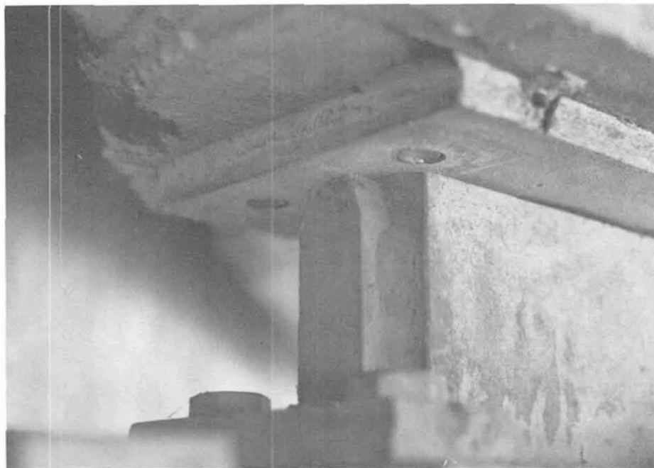
Fig. 5.8 Close-up of rocker bearing showing remnants of sheared keeper plate bolts at top.
