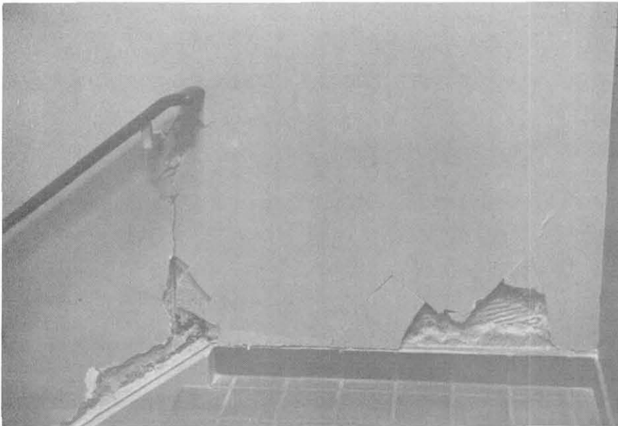
Fig. 8.7 Cracks in plaster wall of Santa Barbara County Administration Building.
