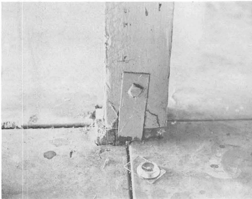
Fig. 7.49 Wood column shifted north in single story commercial building at the Santa Barbara Municipal Airport.
