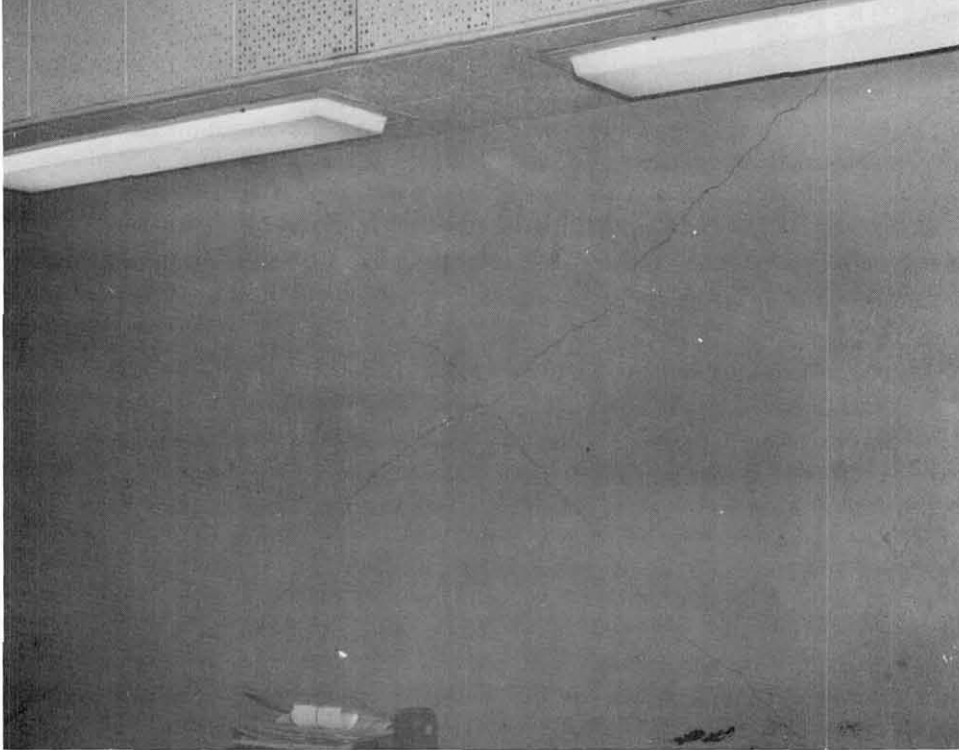
Fig. 7.39 Pattern of X cracks in 10 inch thick R/C shear wall at east end of first story of Administration Building, Delco Electronics facilities.
