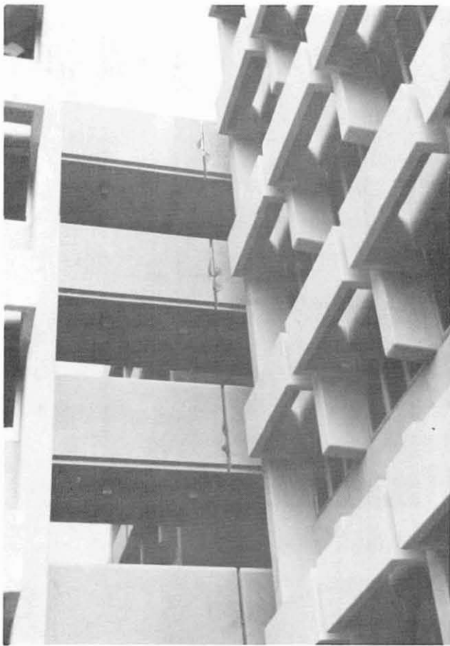
Fig. 11.5 Damage to seismic joints on third through sixth floor walkways between South Hall and the Graduate Tower, UCSB campus.
