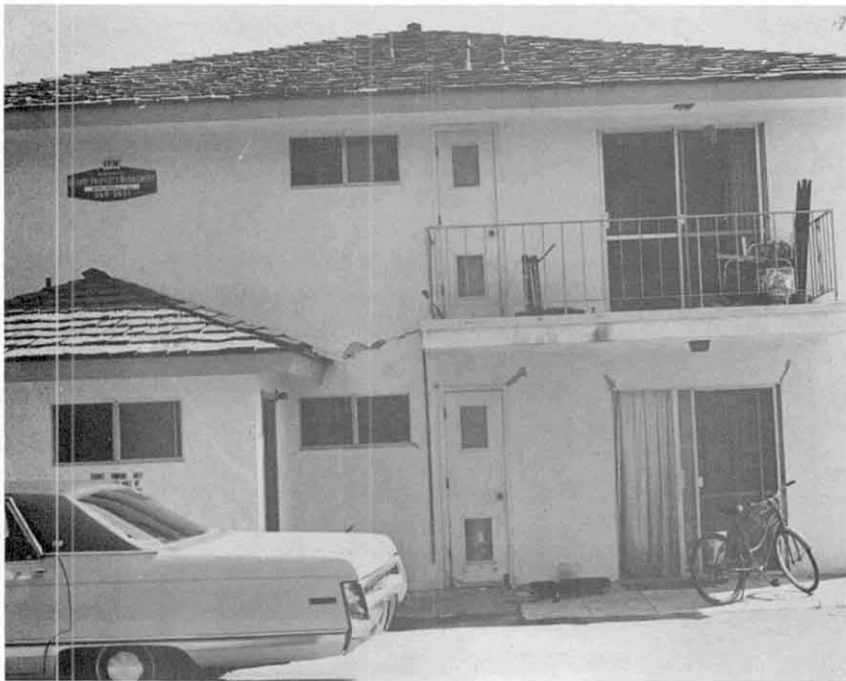
Fig. 7.51 Cracks in exterior plaster walls of two story residential building in Isla Vista.
