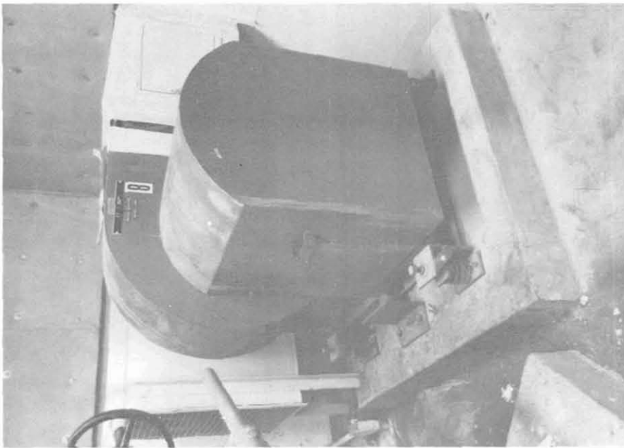
Fig. 8.20 Fan in basement of four-story Library IV Building, UCSB. Vibration supports were not damaged.
