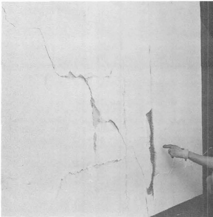
Fig. 7.21 More diagonal cracks in north-south shear walls in first story of Anacapa Residence Hall.
