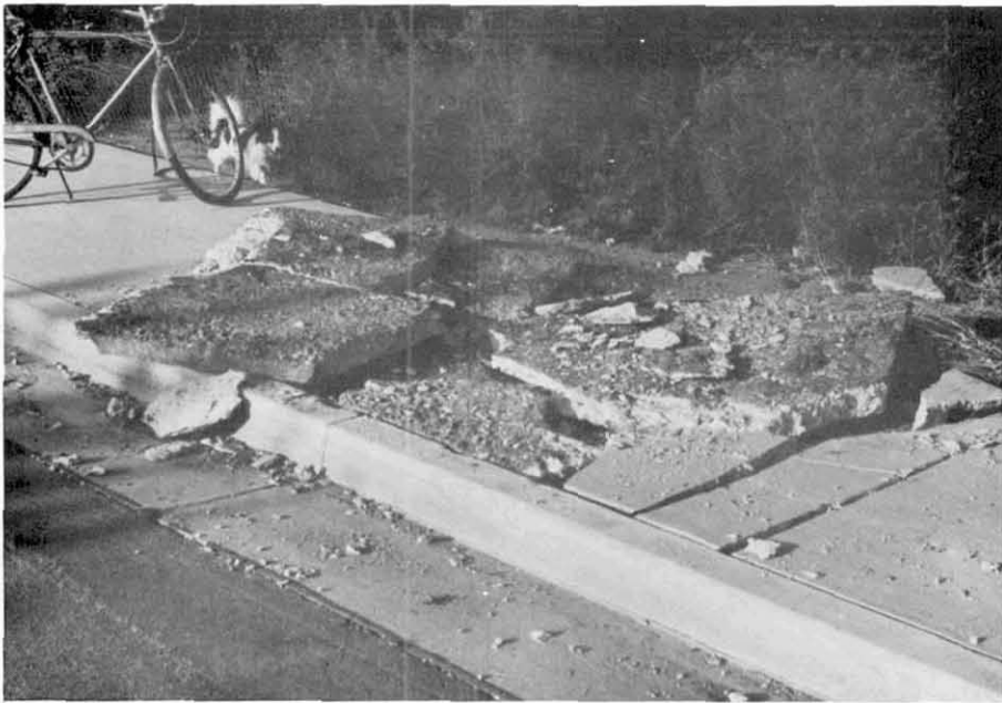
Fig. 9.7 Concrete sidewalk which buckled and fell upside down on Los Carneros Road north of Hollister Avenue, Adjacent pavement, curb, and gutter were not disturbed.
