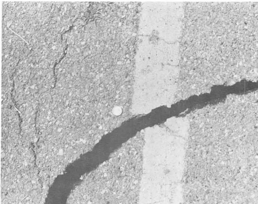
Fig. 9.2 Close up of extension fracture shown in Fig. 9.1. Scale given by the coin (quarter) in the center of the picture.
