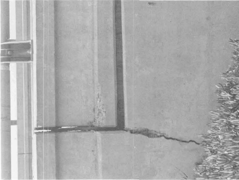
Fig. 5.11 View looking west at joint shown in Fig. 5.10. Vertical crack is on line with face of abutment backwall.
