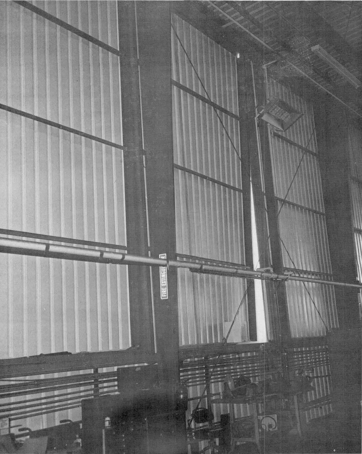
Fig. 7.47 Explosion panel which broke loose at the corner during the earthquake, Flight Physics Laboratory, Delco Electronics facilities.
