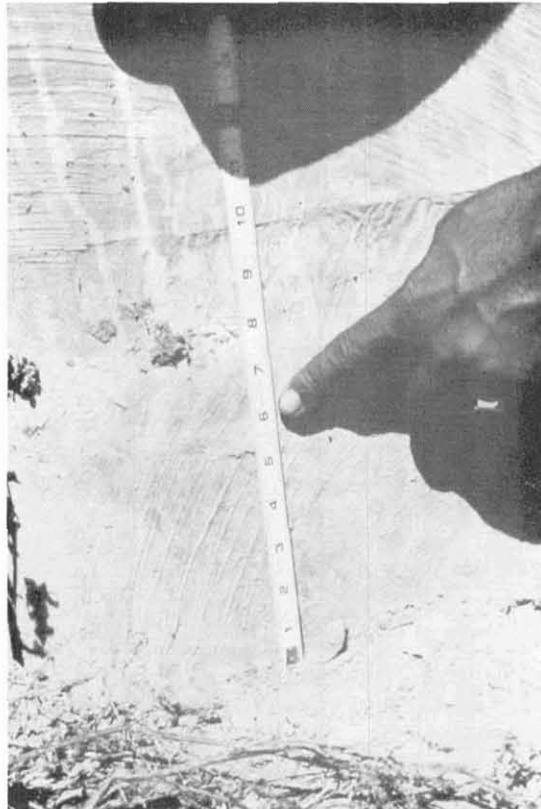
Fig. 9.6 Close up of soil settlement shown in Fig. 9.5.
