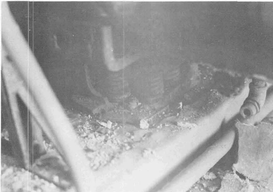
Fig. 8.9 Close up of damaged supports at front of chiller (Fig. 8.8).
