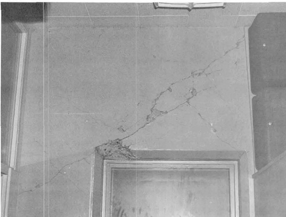
Fig. 7.42 Cracks in shear wall over doorway at west end in first story of Administration Building, Delco Electronics facilities.
