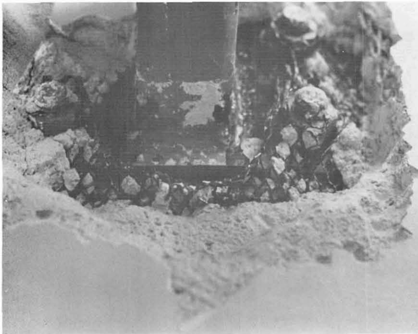
Figure 7.63 View from under bracing tube of damaged joint shown in Fig. 7.62. Note gap between column and bottom edge of connection plate
