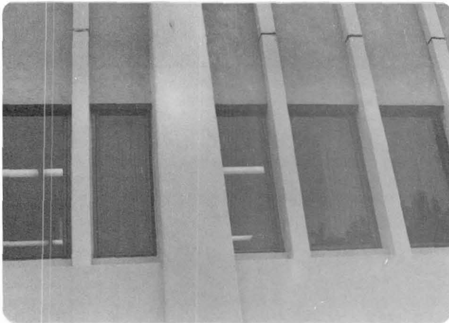
Fig. 7.2 Shear crack forming an X pattern in column in second story of Santa Barbara County Administration Building.
