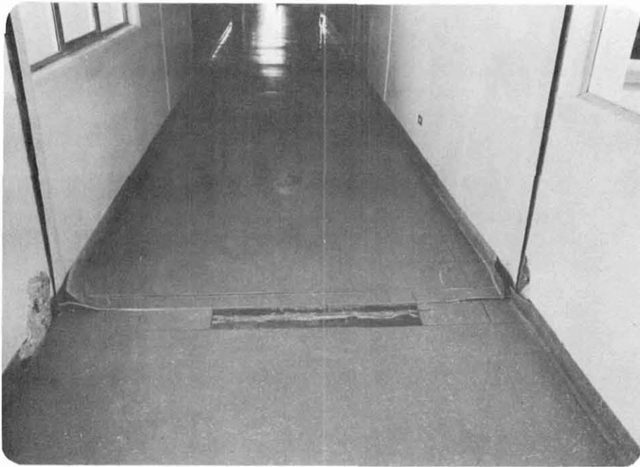
Fig. 11.3 Another damaged seismic joint in South Hall, UCSB.
