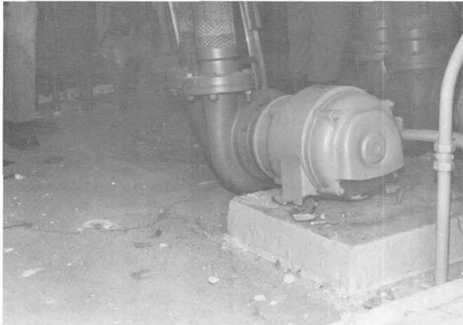
Fig. 8.11 Broken mounting base of hot water pump on top of Library III Building, UCSB.
