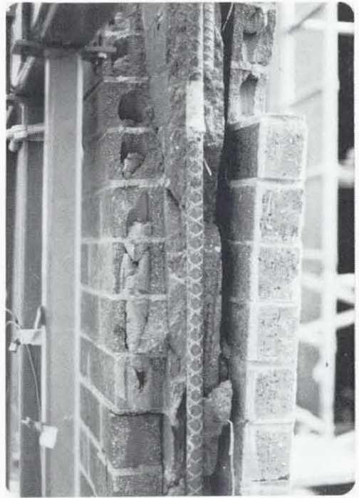
(b) CORE SPLIT IN GROUDED CORE BRICK WALLS
