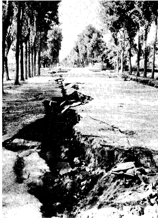
FIGURE 4.63 Damage to a road caused by soil failure.
