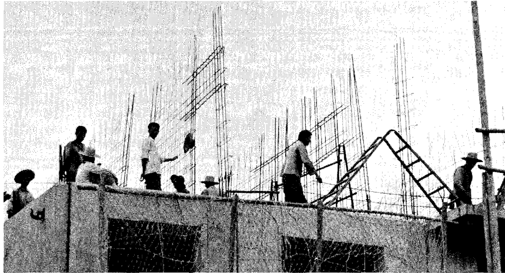
FIGURE 3.19 With one cycle completed, reinforcing for transverse shear walls is placed. Building is that shown in Figure 3.17.
