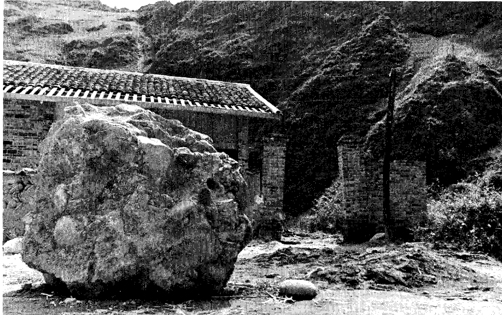
FIGURE 5.16 Large conglomerate boulder that fell during the SP earthquakes. Note also the structural damage to the building.
