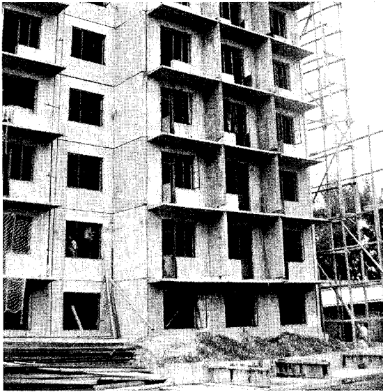
FIGURE 3.14 Exterior view of typical apartment building in Peking. The building has precast exterior walls, precast floors with topping, cast-in-place concrete shear walls, and brick partitions.
