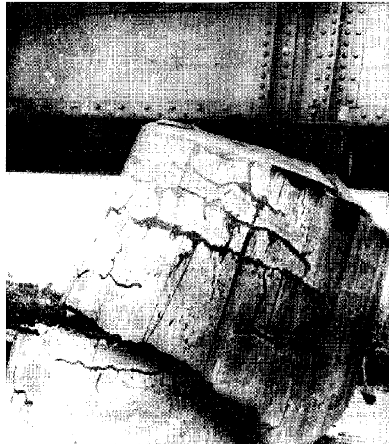
FIGURE 4.59 Broken pier of railway bridge 55 on the Peking-Shanhaikuan line.
