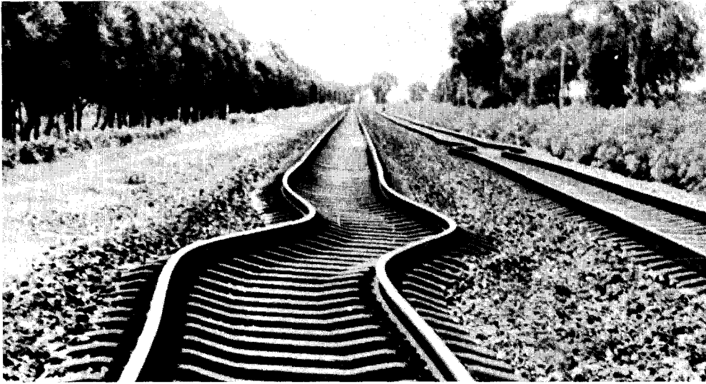
FIGURE 4.3 Buckling of rail lines due to ground deformations. The general Tangshan region had many soft soils that behaved poorly during the earthquake.
