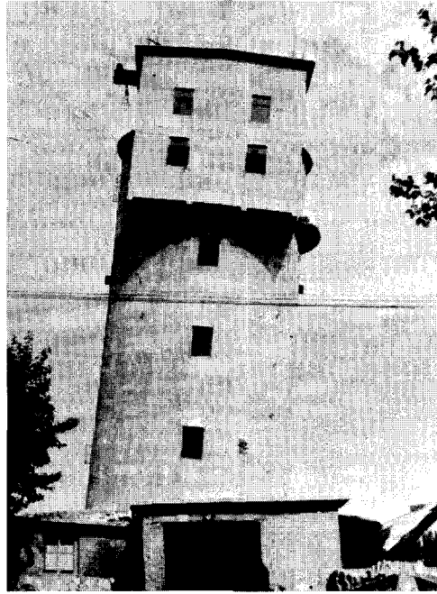
FIGURE 4.42 Tilted ventilation tower at Tangshan coal mine.
