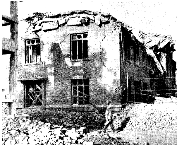
FIGURE 4.46 Partly collapsed five-story building at Coal Mine Design Institute in Tangshan.
