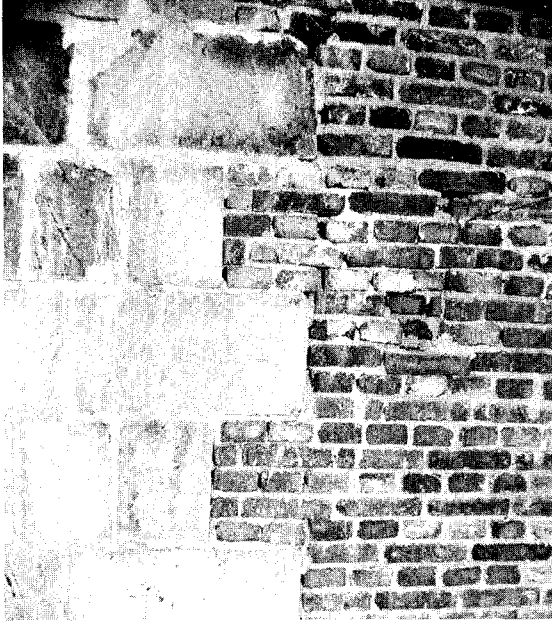
FIGURE 3.29 Harbin apartment building of Figure 3.28. Some of the interior brick walls are meshed with exterior block walls.
