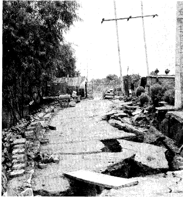
FIGURE 4.5 Damage to road near Loting Hsien. Slumping, lurching, and settlement of soft soils caused extensive damage to highways in the Tangshan region.
