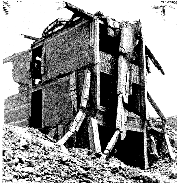
FIGURE 4.29 Collapsed five-story office building, Tangshan. The lower three stories had concrete columns, and the upper two stories were unreinforced brick without concrete columns.
