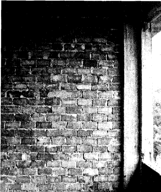
FIGURE 3.45 Transverse brick shear wall made with bricks similar to those shown in Figure 3.34, Chengtu office and storage building.
