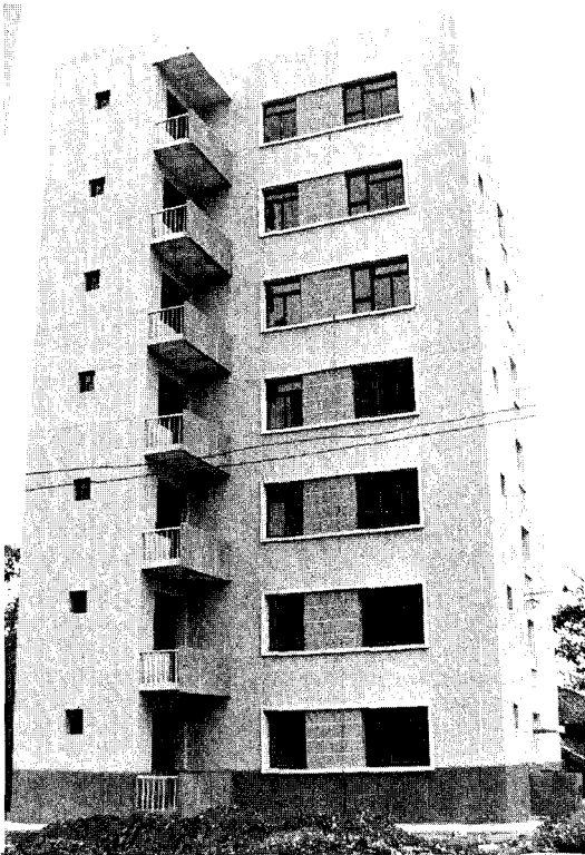
FIGURE 3.33 Nearly completed seven-story apartment building in Chengtu. The building has brick bearing walls and precast concrete floor slabs.
