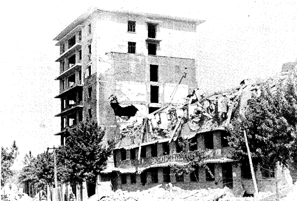
FIGURE 4.32 Eight-story Hsinhua Hotel in Tangshan was badly damaged at the fifth-story level but remained standing. In the foreground is a collapsed six-story building.
