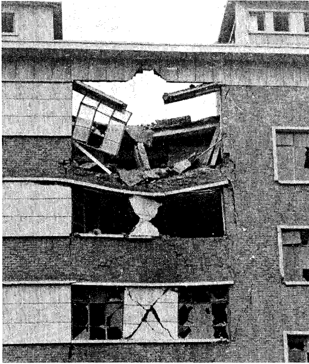
FIGURE 4.49 Damaged reception building in Tangshan.
