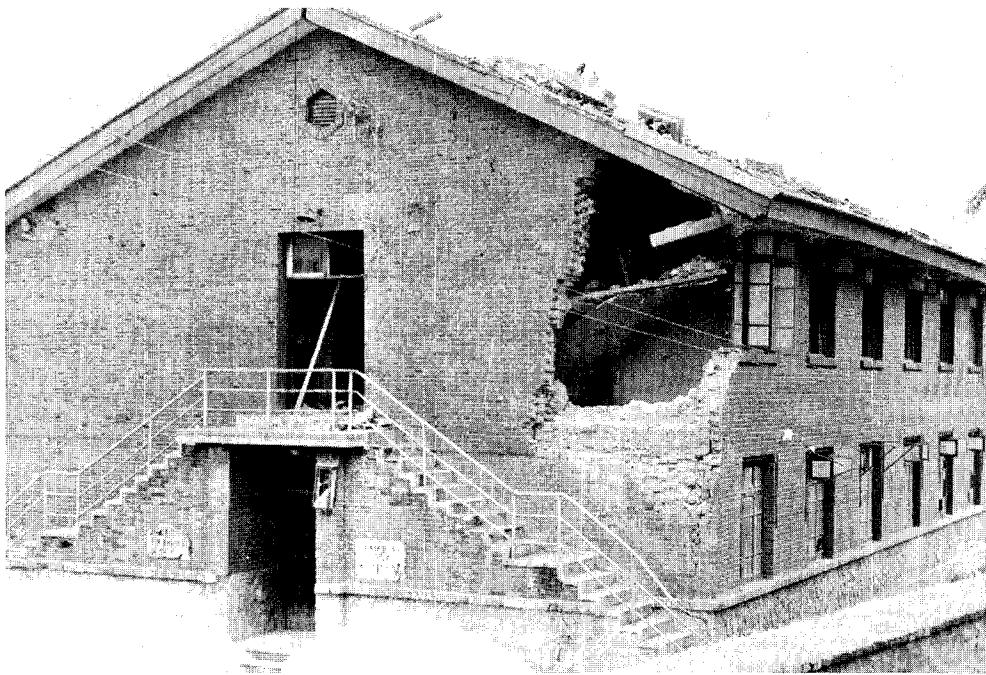
FIGURE 4.50 Damaged Tangshan second reception building. Although damaged, this two-story brick building remained standing.
