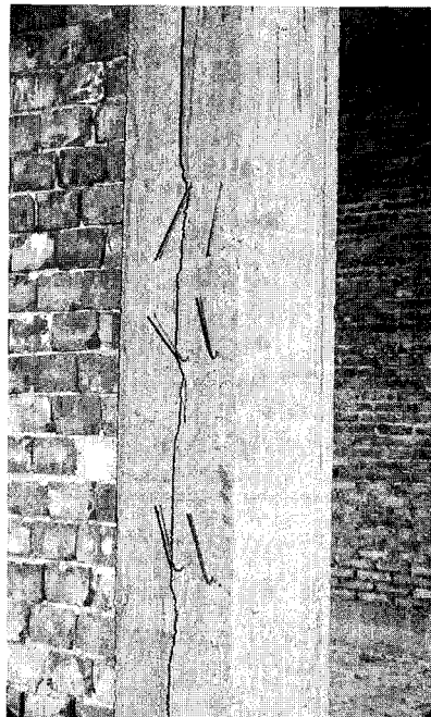
FIGURE 3.46 Brick shear walls in the Chengtu office and storage building had dowels protruding from adjacent columns, but shear keys were not provided.
