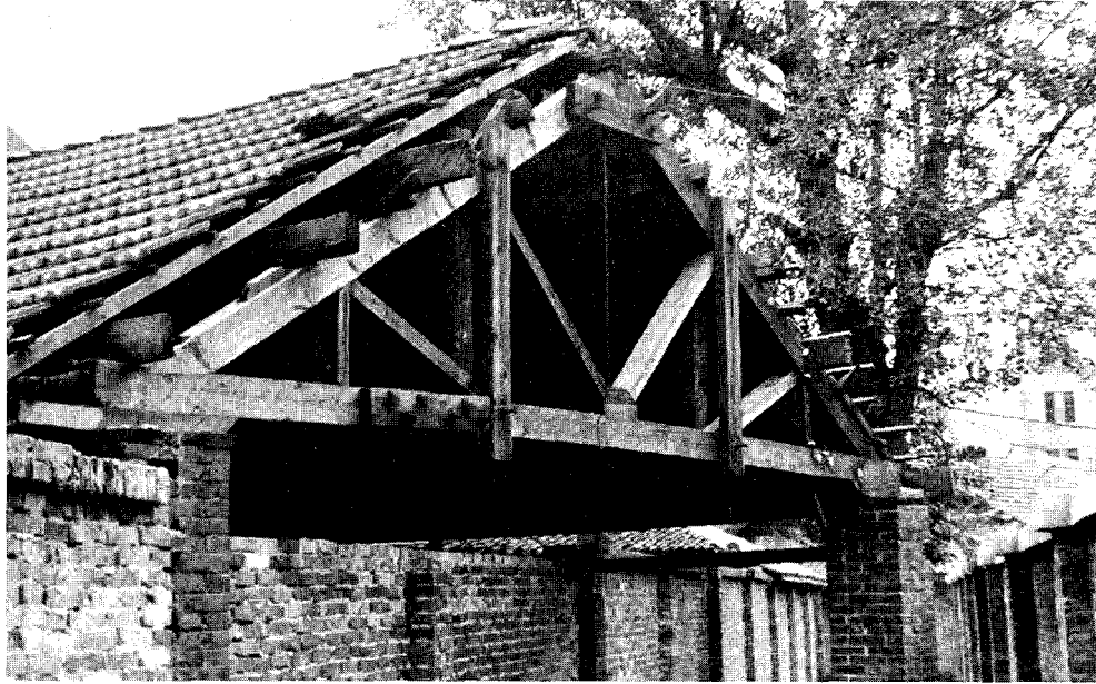
FIGURE 3.35 Timber truss on small building in Chengtu near apartment building of Figure 3.33. Note unreinforced brick columns, which are used extensively in China.
