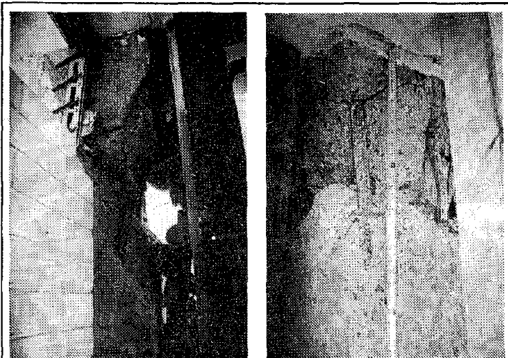
FIG. B3.1 CAPTIVE COLUMN SHEAR FAILURE (Column "54")
