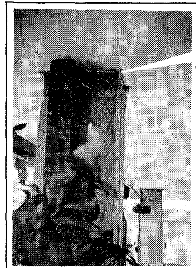
FIG. B3.2 BENDING FAILURE AT COLUMN TOP
