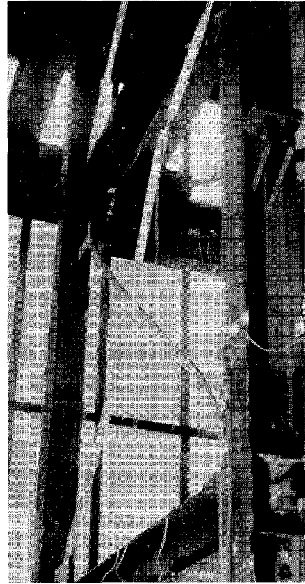
2nd Floor Buckled Pipe
