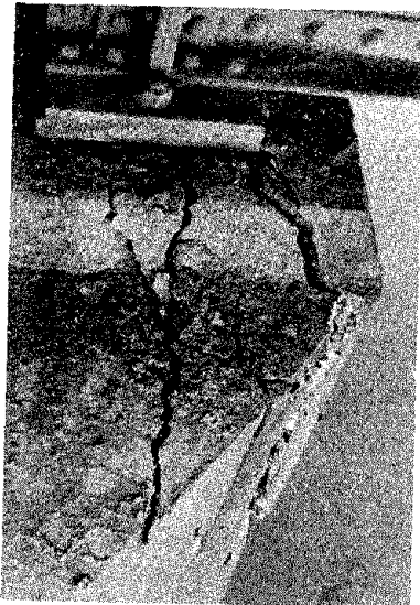
Fig.32 Failure of Concrete near a Bearing, Kimazuka Bridge
