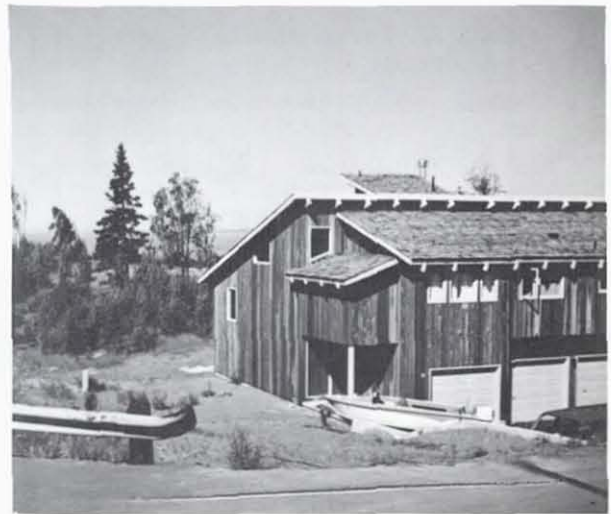
Figure 32. Duplex under construction at end of McKenzie Drive on the Turnagain landslide, Summer 1978. See Figure 27 for location.
