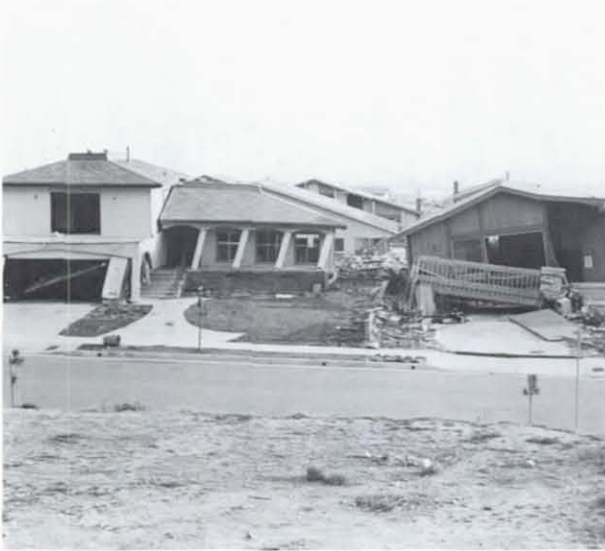
Figure 14. Two severely damaged split-level houses (Source: Jennings, P.C., ed., 1971, p. 289)
