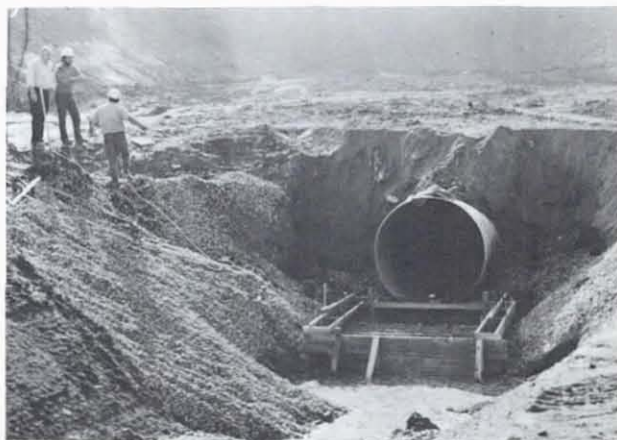
Figure 15. Storm drain installed in channel at the bottom of Bluebird Canyon, December 1978
