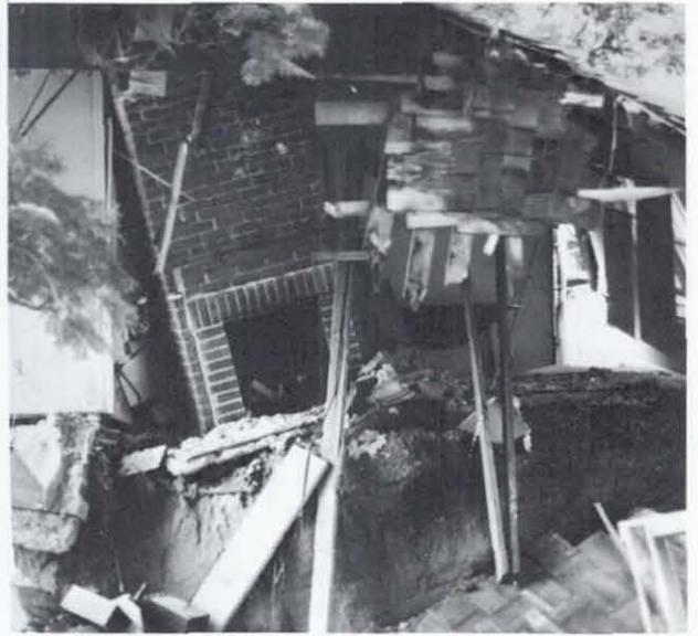
Figure 10. Interior of house shown in Figure 9, October 5, 1978
