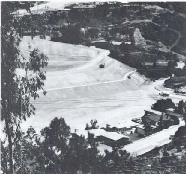
Figure 19. Landslide area with buttressing essentially complete and rough grading for roads and utilities underway, July 1979
