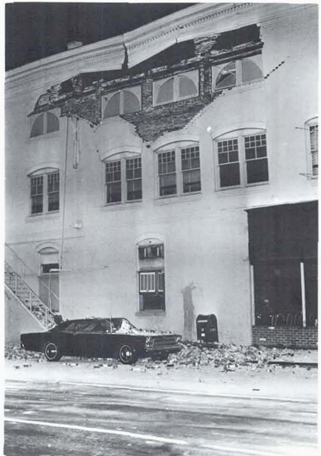
Figure 4. Unreinforced brick masonry failure, Third Street at Mendocino Avenue.
