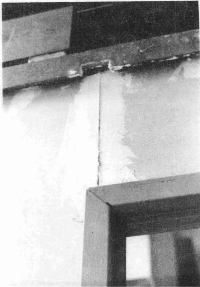
Fig. 88: Partition Test Specimen P11: Failure Above Door Opening
