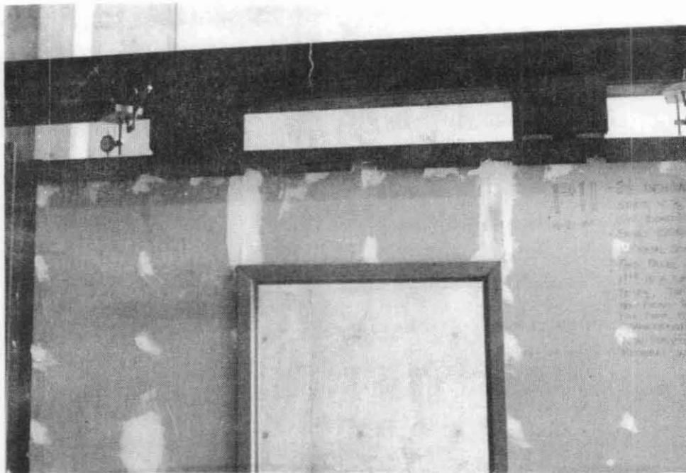
Fig. 85: Partition Test Specimen P11: Failure Above Metal Door Frame Opening
