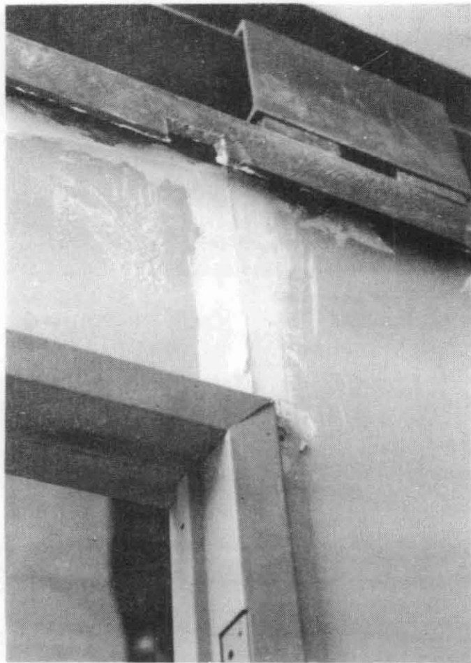
Fig. 91: Partition Test Specimen P11: Failure Above Door Opening
