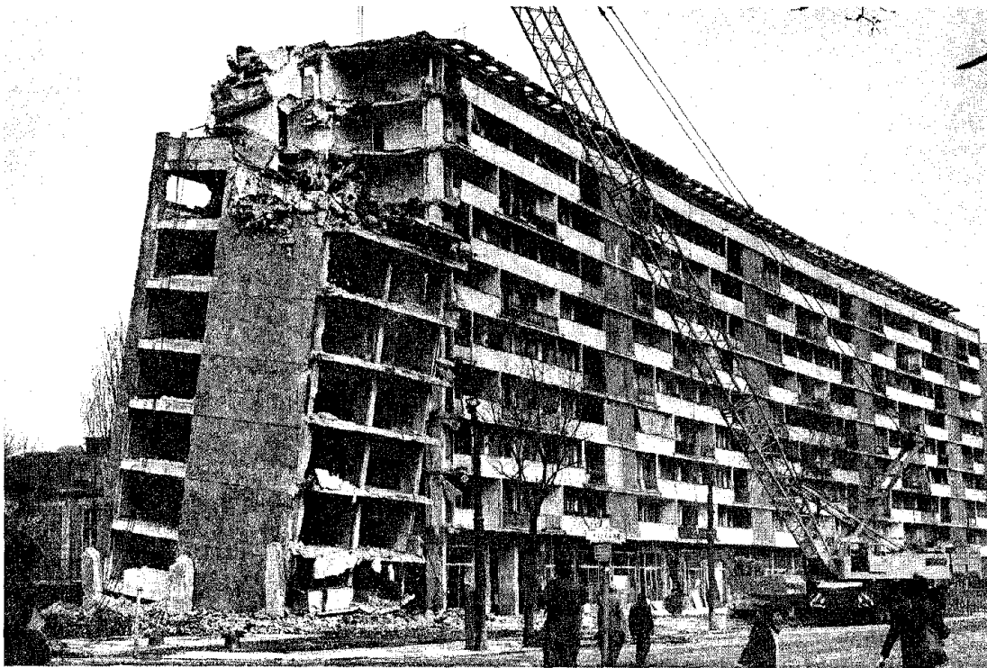
Figure 19 Partial collapse of new apartment building.
