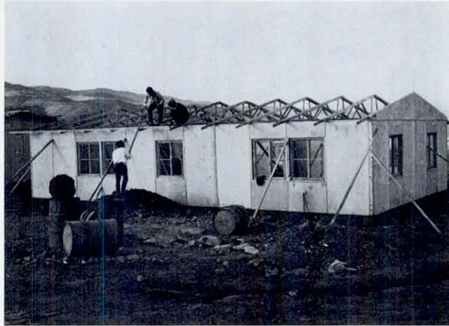
FIGURE 86 Buildings in Bingöl of prefabricated wall panels and roof trusses to be used as offices for resettlement construction. The walls consist of a 3-cm exterior layer of cement-asbestos, 5-cm of fiber glass, and an interior surface of 1-cm wood chip board. The walls are attached to a concrete floor slab by bolting to punched galvanized steel angles. This type of building has been suggested as housing for villagers, but it is doubtful if it would prove warm enough for Bingöl's cold winters (sometimes as low as -30^{\circ}\text{C} ) or sturdy enough to stand up under the rough usage conditions of village life.
