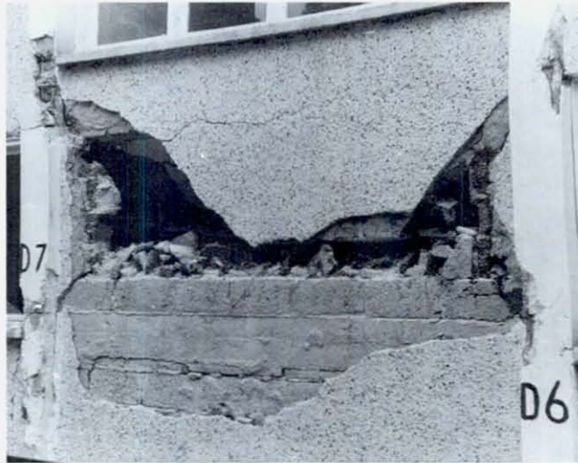
FIGURE 63 Column damage in the rear of the hospital. Most columns fractured at the top and bottom of window openings, being relatively fixed by concrete spandrels and cinder block walls above and below these openings.
