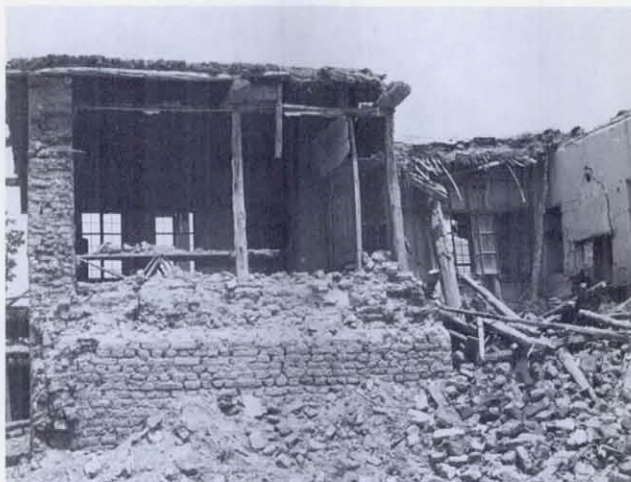
FIGURE 15 A lesson concerning adobe house construction is illustrated in this figure. The roof is at least partially supported by wood columns, and although the front wall collapsed, the roof did not.
