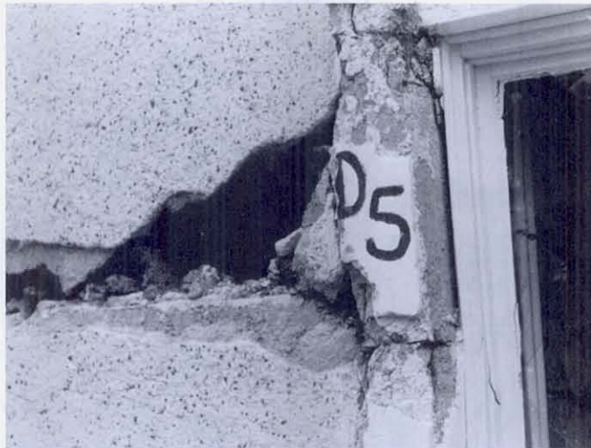
FIGURE 64 A close-up of column damage at the rear of the hospital. Concrete was rather soft to a knife point, but no honeycomb was evident. The small column dimensions in the longitudinal direction of the building raise the suspicion that earthquake forces in the longitudinal direction were not considered in the design.
