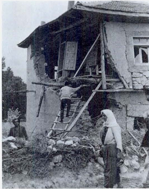
FIGURE 17 Temporary wood braces have been installed to prevent further collapse of this adobe house in Yaziköy, Burdur. In the second story the side wall and the front wall appear to have had no connection. First story walls are probably tied to each other only with interlaced adobe bricks. Is there a relationship between failure of the lower corner and failure of the second story side wall? (Photograph courtesy of Prof. Asim Yeginobali)
