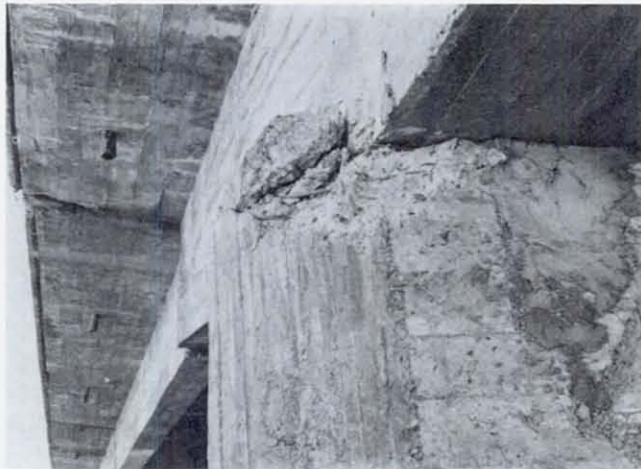
FIGURE 82 A close-up of damage at the top of the westmost pier. Note the poor placement of concrete and the patching. Diagonal steel extending into the shoulder at the top of the pier would have increased its strength.
