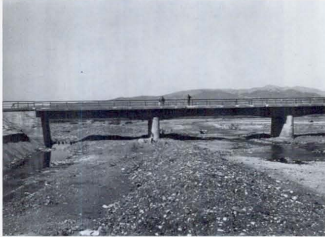
FIGURE 78 Looking south at one half of the 5-span concrete bridge across the Göynük River at Köprübaşı, 10 km east of Bingöl. An extension of the line of the 8 km earth crack in the Göynük River bottom passes near here, but no crack was actually observed at this location. The center span and the end span both are continuous across their piers to support a simple span in the second bay from the abutment, the joints of which are visible at deck level. Pier spacing is about 24 meters.
