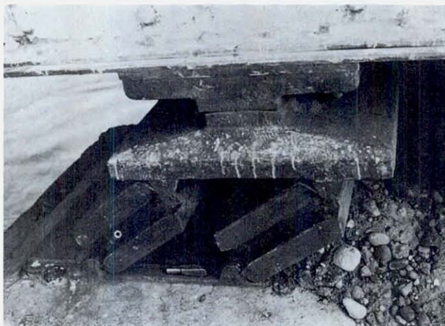
FIGURE 74 Rocker supports on the west end of span No. 3. This pier (No. 2) apparently shifted to the left (east) by about 15 cm, causing the relative displacement shown. The rockers did not fall completely because of restraining knobs on the base plate, but are obviously not now supporting the span. It is probably supported by interference of the bridge structure with span No. 2. The fixed support of the east end of span No. 2 pulled it to the east when the pier shifted, causing the railing to buckle (next figure) and pulling the span completely off its rocker support on pier No. 1. Sideways movement of some 20 cm of span No. 2 permitted the rockers to slide completely off the base plate on pier No. 1, dropping the end of the span 22 cm. The knife in the figure is 8.5 cm long. The need for bridge bearings which can accommodate pier displacements is obvious.
