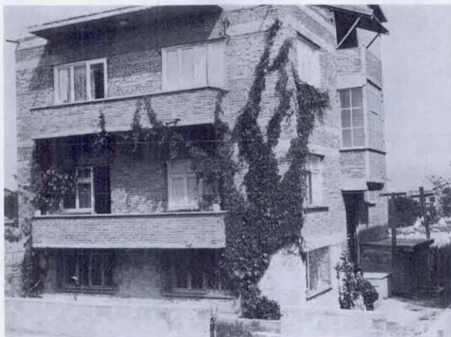
FIGURE 36 Next door to the building with shattered foundations in the previous figure stands this structure which had only minor cracks between foundation stones. The two buildings differ in that this is one story less, and its foundation is made of hard stone. Did the stone or the extra story make the difference in damage?
