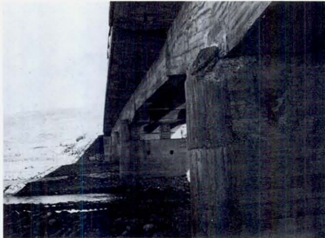
FIGURE 79 The south side of the bridge, showing lateral movement of the simple span relative to the adjacent continuous spans, and failure at the tops of the piers due to sideways force from the superstructure. The nearest pier here is the left-most pier in the previous figure.
