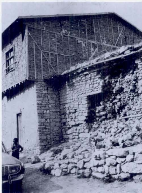
FIGURE 24 In the village of Kisla, near Burdur, a region of light shaking, the face of a stone wall laid in mud mortar has fallen due to lack of long stones to tie the faces together. This mode of failure is not uncommon in thick stone walls. Next door the lightly braced second story of poorly laid brick appears to have lost one triangular panel of brick. As flimsy as it is, the wood framing probably supports the roof, but the brick walls contribute the greatest amount to earthquake load.
