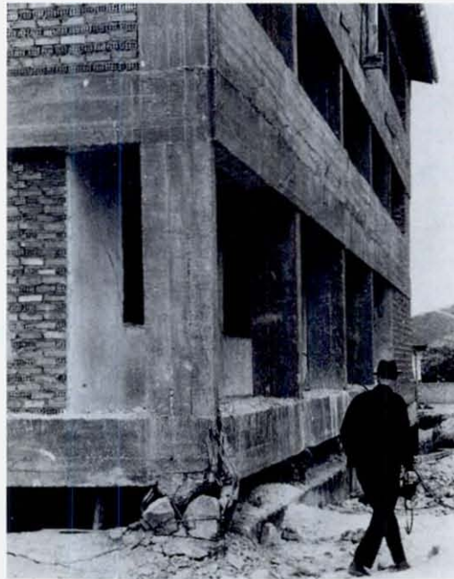
FIGURE 67 A close-up showing shattered columns, and some cracking of brickwork. Interior columns in the basement were free to deflect over their entire height, whereas the exterior columns were greatly restrained by the heavy basement walls. This great difference in stiffness resulted in all the lateral load being resisted by the exterior columns, and consequently suffering all the damage. Note that the columns are weaker in the longitudinal direction of the building, but column damage appears to be caused chiefly by motions in the transverse direction. Plans and additional photographs of this building are shown in Reference 12. (Photograph courtesy of Prof. Asim Yeginobali)
