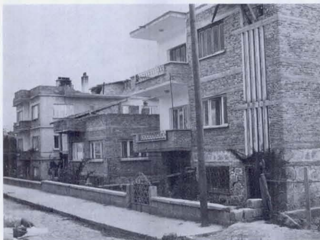
FIGURE 37 The situation pictured here is similar to that illustrated in the two previous figures. The buildings on the ends have travertine foundations, and are badly cracked (see the following figure), but the building in the center, one story shorter, has a foundation of hard stone - limestone or a very fine-grained sandstone - and it suffered no cracks at all. In this neighborhood of Burdur there was great variation in damage, even among buildings with travertine foundations.
