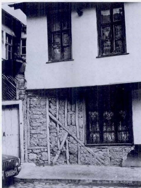
FIGURE 40 An older structure in Burdur, from which the plaster cracked. The bracing is not ideal, and the lack of continuity of the columns shows ignorance of structural principles, yet the construction is much better than plain adobe. The use of brick or adobe infill in braced wood frames as insulation and plaster base is common in older structures. This type of construction would have much merit if proper framing was used with hollow inexpensive bricks.
