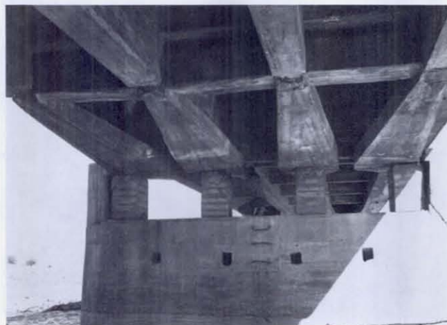
FIGURE 80 Damage to the second pier from the west abutment and to the junction of the simple span with the central continuous span. The cause of the large crack near the bottom of the pier is not known.
