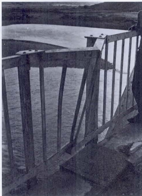
FIGURE 76 Looking downstream (south) at the buckled railing, span No. 3 on the left, span No. 2 on the right. Span No. 2 was dragged into span No. 3, which is fixed to the east abutment, by the shifting of the pier below.
