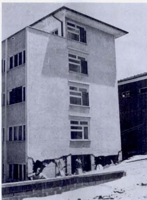
FIGURE 61 A closer view of the south end wall of the hospital showing the columns to be relatively weaker in the longitudinal direction of the building. The furthest corner is completely fractured, and has begun to fall away from the structure.
