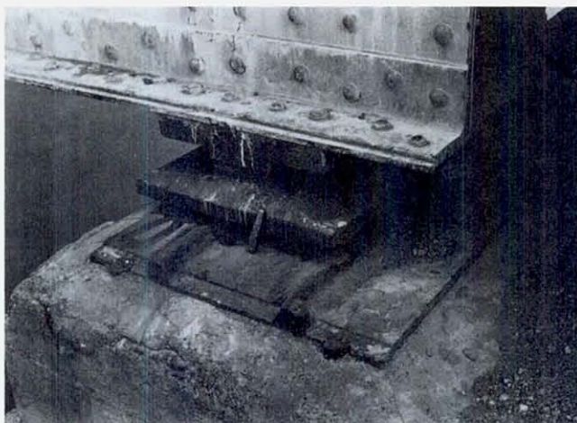
FIGURE 75 The west end of span No. 2 on top of pier No. 1, looking downstream. Sideways displacement of the span permitted the rockers to fall completely off the pier, dropping the span 22 cm vertically onto its base plate. The displacement here is about 20 cm downstream and 12 cm to the east.
