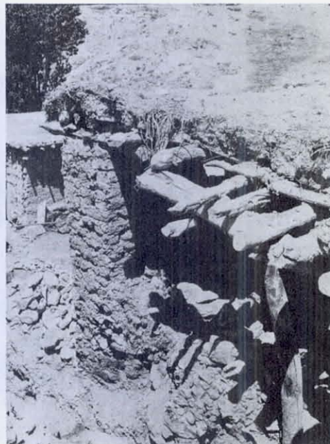
FIGURE 21 Showing the construction of a mud roof on an adobe house. Successive layers of logs and poles, at progressively closer spacing, support finally twigs and leaves, with mud on top. More mud is added over the years to keep the roof watertight.
