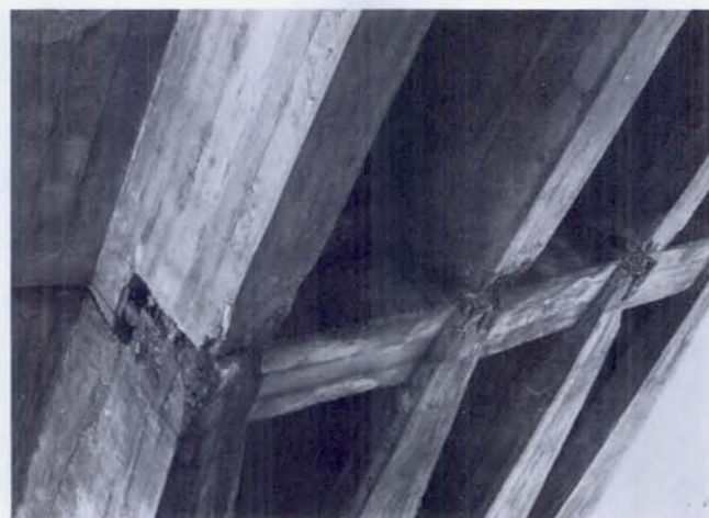
FIGURE 81 Damage to the south roller support for the simple span, which rests on the overhang of the central continuous span. Only the two outer girders carry the reaction. The beam which distributes the loads from the inner girders to the outer girders can be seen faintly under the deck. Note the concrete cracking in the overhanging lip of the simple span.
