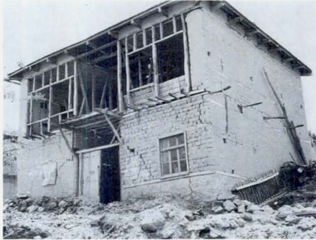
FIGURE 22 This house under construction in Yaziköy, Burdur, has diagonal bracing in upper interior walls, but none in the front wall. Perhaps the hip roof, a rather rigid construction, held the second story walls together. First story adobe walls, without diagonal bracing, are heavily cracked. Mud plaster covers the adobe on the left side.
