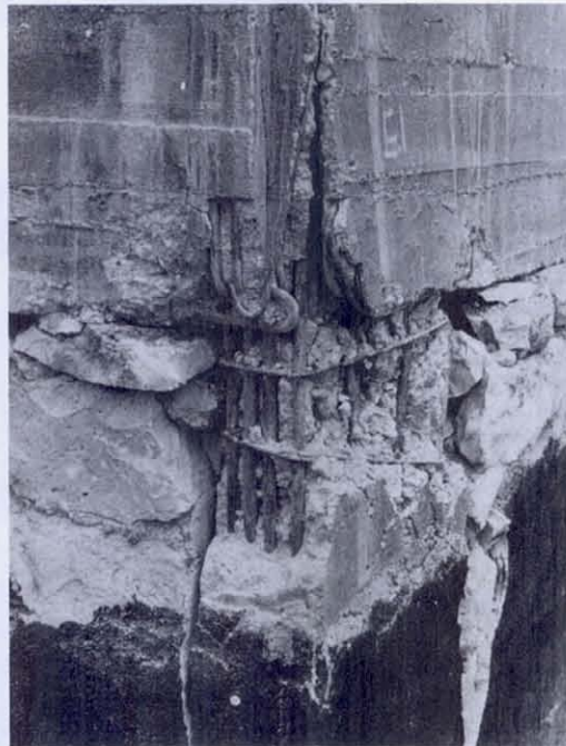
FIGURE 69 Another corner column at the top of the foundation wall in the new Burdur school: heavy beams not tied together, permitting concrete to be lost; a laterally weak column insufficiently tied; and poorly compacted concrete. A designer might have assumed that the foundation walls would brace the column and prevent failure, but the walls are of no help against forces directed toward the outside. In hindsight, a better design would be to rest the first floor slab directly on the foundation walls, providing a large area for the transfer of horizontal forces. (Photograph courtesy of Prof. Asim Yeginobali)
