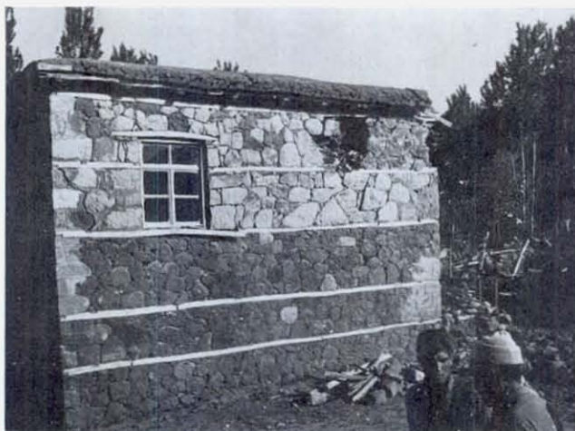
FIGURE 27 The beginning of disintegration of a stone, mud-mortar house in Ekinyolu. Note the corner cracks, perhaps inhibited by the wood bond members, and the falling out of the outside face of the wall near the roof. Under continued shaking the upper part of the wall would likely disintegrate, allowing the roof to fall in.
