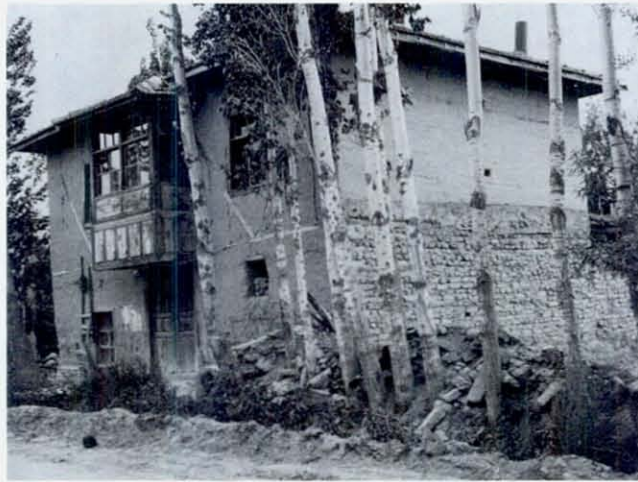
FIGURE 23 This two-story adobe house in Yaziköy, 20 km SW of Burdur, survived, although 193 out of 250 houses in the village collapsed or were heavily damaged. Poplar trees, as seen here, are commonly planted in the villages for fuel and lumber. Increased plantings of poplars and proper instruction for their use in building braced frames in houses would reduce earthquake fatalities.
