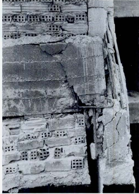
FIGURE 70 Another corner column in Burdur's new school building, across from the hospital. Would bars in the spandrel beams extending around the corner have prevented this failure, or would such additional reinforcement simply lower the point of failure to just below the beams? (Photograph courtesy of Prof. A. Yeginobali)
