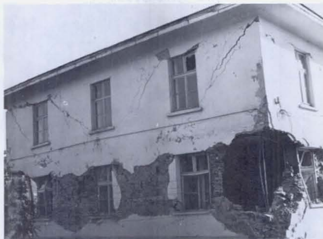
FIGURE 32 End view of a damaged wing of the government building in Bingöl. Cracking in second stories was unusual in Bingöl. Note the cracks seem to start (are widest) at the corners of the building, at the top, where dead load compression is least. Cracks of x-shape occurred in the first story, but cracks were only in one direction in the second story. Perhaps under continued shaking, x-cracking would have occurred in the upper story, resulting in the upper corner dropping out.
