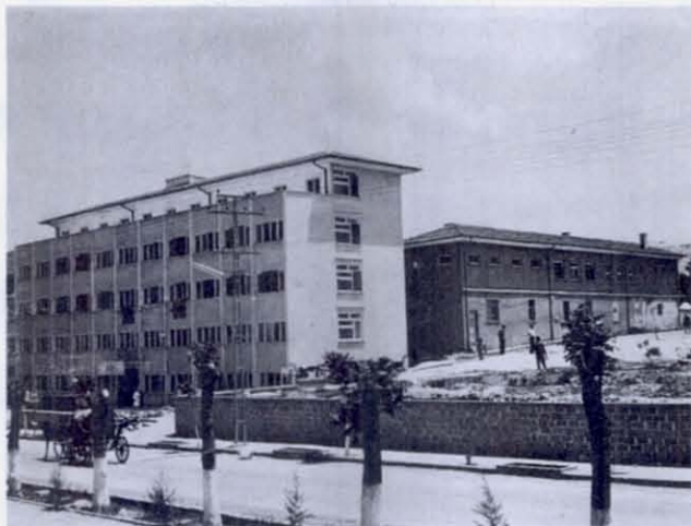
FIGURE 60 Burdur's new 5-story reinforced concrete hospital had every column in the first story broken in flexure, leaving the building slightly displaced in the longitudinal direction. The two-story reinforced concrete framed laundry building, on the right, had only minor masonry cracking on one end wall. No damage was observed on the concrete block wall in the foreground.
