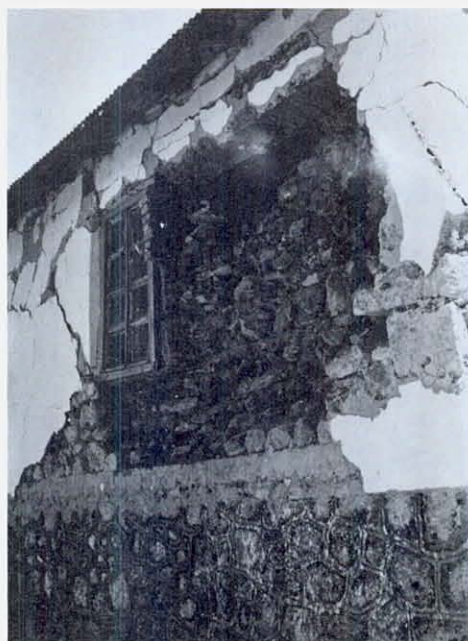
FIGURE 31 The foundation of the 1\frac{1}{2} -story school in Hacilar, in the Bingöl district, was laid in hard cement mortar, but upper walls were of rubble laid in weak mortar. Above the windows were a reinforced concrete collar beam and a roof of corrugated steel. No foundation damage was evident, but the rubble walls simply fell apart in places. The weakness of walls made of small stones which do not extend completely through the walls, laid in poor mortar, is obvious.
