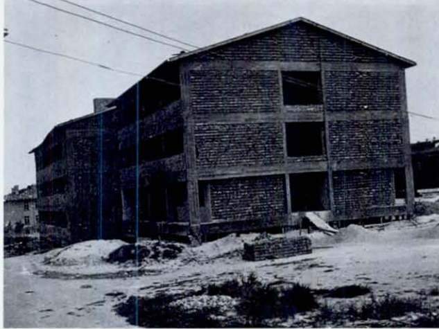
FIGURE 66 Under construction, across the street from Burdur's hospital, is this 3-story school, of rather common design in Turkey. Every exterior column, between the top of the foundation wall and the bottom of the first floor, was shattered, causing the building to settle slightly. There was also minor damage to brickwork at roof level and in the first story. Note the chimneys standing in the background.
