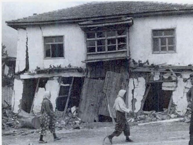
FIGURE 18 This two-story adobe house, on the verge of collapse, contains lateral bracing in the first story. The 60-cm thick walls with wood posts around the windows appeared very strong to the builder, but proved quite inadequate under lateral loading. The front wall in the second story, probably braced like the house in Figure 17, remained rigid, but could not save the building. (Photograph courtesy of Prof. Asim Yeginobali)
