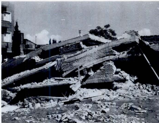
FIGURE 39 Seven persons were killed in the collapse of this 3\frac{1}{2} -story masonry apartment building in Burdur. Mortar was made from lime and sand, and travertine was used in the exterior wall, in the lower story. Possibly the walls of the lower story disintegrated unevenly, causing the building to tilt, thereby increasing the shear force on the walls of the upper stories to the point of failure. This building, on a corner lot, was the only collapsed structure for several city blocks. Others in the immediate vicinity suffered cracked lower story walls, but not to the point of disintegration. (Photograph courtesy of Prof. Asim Yeginobali)
