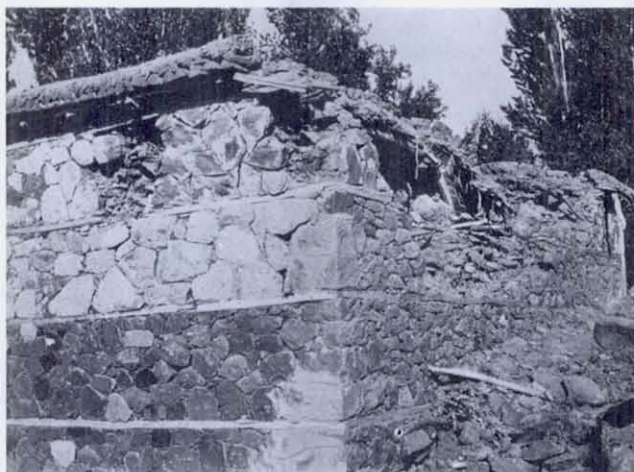
FIGURE 28 Another example of the early stages of failure of a stone, mud-mortar wall - falling out of the outer surface and collapse of the upper portion of the wall which is not tied by the roof beams. There is also some corner cracking.
