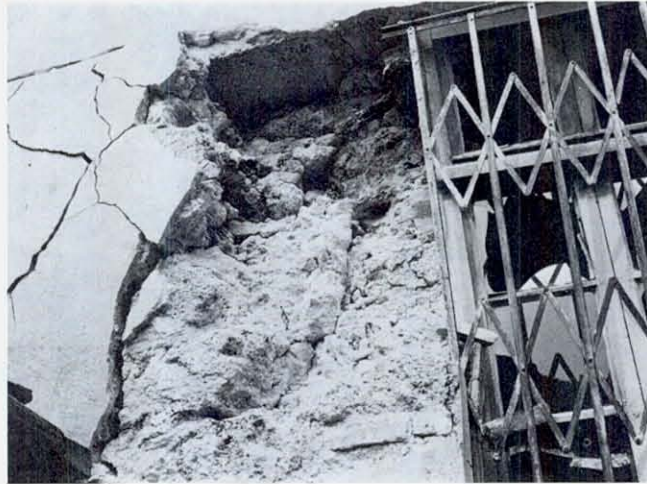
FIGURE 34 A close-up of a shattered travertine foundation wall in Burdur. The stones vary in quality, but usually they contain bands of fibrous or porous material, easily penetrated with a knife. Mortar is probably weakened by the absorption of moisture into the porous stone.
