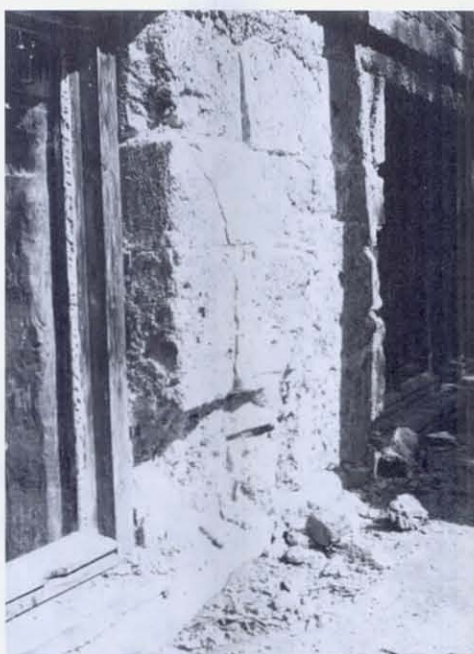
FIGURE 33 The foundation walls of most of Burdur's apartment buildings are made of a porous travertine, consisting of rather hard shelled tubules, randomly spaced, with softer material, almost like rotten bone, between the tubules. The Turkish name for the stone, mined a short distance SE of Burdur, is "Kurna." Here the author has easily thrust his pocketknife, not into a joint or a crack, but into the solid stone itself.
