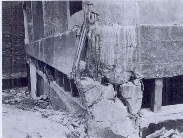
FIGURE 68 A close-up of the nearest corner column appearing in Figure 66. Additional column ties, more strongly anchored - perhaps by welding, would have been required to prevent this failure.
