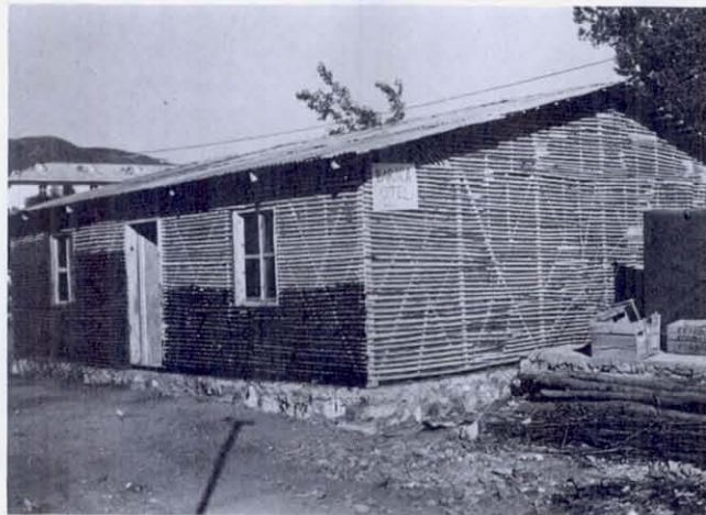
FIGURE 93 This structure, erected in Bingöl after the earthquake, suggests a possible construction type for villagers and others who build their own homes. The columns are 10-cm square, and insulation consists of small pieces of mud poured into the wall voids as the lath application proceeded upward. Plastered inside and out, this structure would be weathertight, moderately warm, and safe during an earthquake. The major cash outlays would be for nails, corrugated steel roofing, and the sawing of the lumber.
