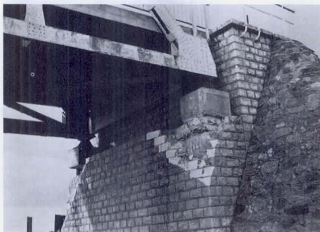
FIGURE 77 The east abutment, showing the end of span No. 3. The facing stone has been broken away to permit inspection of the structural damage. The horizontal failure plane in the concrete appears to be a construction joint. Consideration should be given in design to the possibility of construction joints in piers having to withstand lateral as well as vertical forces.
