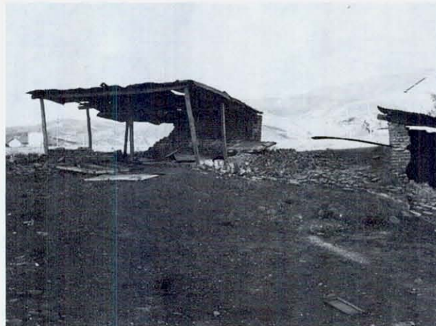
FIGURE 55 This crude shed in Bingöl illustrates a principle. The brick walls collapsed, but the roof, supported on wood columns, even though they were unbraced, did not fall. On the right, not completely shown, a roof supported on only brick walls came down with the walls. Braced frames which could carry roof loads, even though masonry walls fall, would offer considerable added safety in masonry structures.
