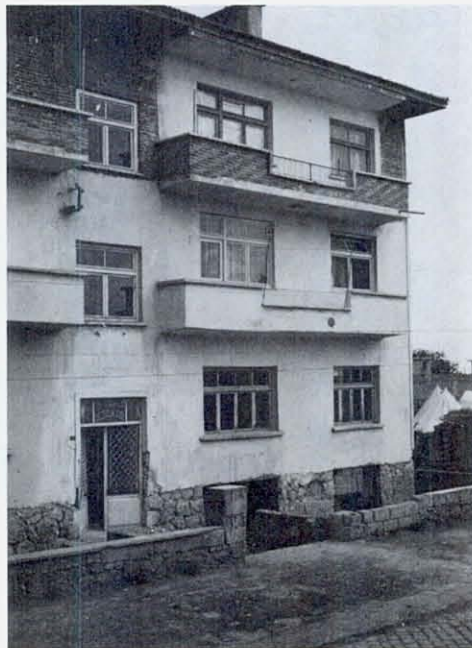
FIGURE 35 This building has been evacuated because the travertine foundation walls are shattered. The next figure shows the building adjacent to this one.
