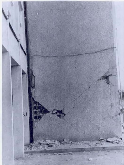
FIGURE 65 The north end wall of the hospital, front wall to the right, with a front column exposed. Note that the diagonal crack in the cinder block wall continues through the column. The outside faces of the cinder blocks have broken off and fallen with the exterior plaster. The white columns on the left support a passageway to an older masonry building.
