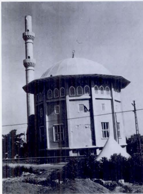
FIGURE 57 Yeni Mosque, just east of the fairgrounds in Burdur, suffered badly cracked cinder block walls between concrete columns, but no damage to major columns. So little cement had been used in the cinder blocks that they could almost be broken in the hand. The undamaged minaret, not yet completed with a cap, should be a model for future minaret construction. Reinforcing steel, just visible at the top, was placed in hollow blocks, which were then filled with mortar. Mortar and bricks observed near the base of the minaret were of good quality.
