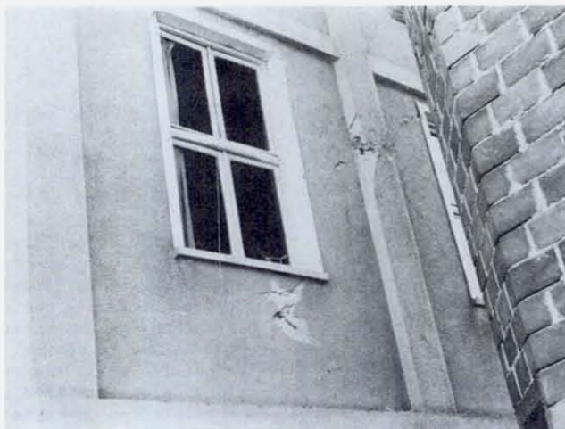
FIGURE 58 When the masonry panel in the entrance structure of Yeni Mosque cracked diagonally, this light reinforced concrete column cracked with it, its stiffness and strength having no noticeable influence on the behavior of the wall. This is in contrast with the performance of the heavy columns supporting the roof, shown in the previous figure.
