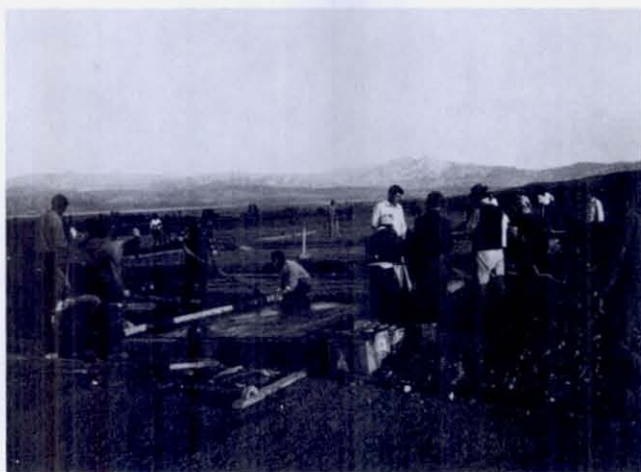
FIGURE 88 Machinery is scarce and manpower plentiful in most of Turkey. Here men mix and place concrete by hand for floors of prefabricated buildings in Bingöl. Laborer's wages were about $1.75 per day at the time of this report.
