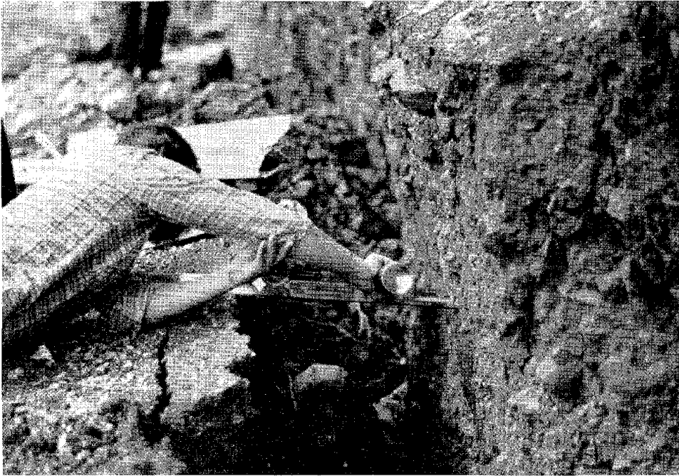
FIGURE 2.12 Typical ground rupture along the Kalamaki and Kapareli traces. At this location there were 60 cm of dip-slip displacement and 50 cm of rotational "opening" displacement.
