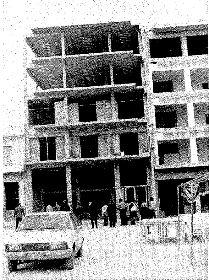
FIGURE 4.17 Flat slab construction without any stiffening walls in Megara. The brick walls were constructed afterward. The building suffered considerable damage with permanent deformations.
