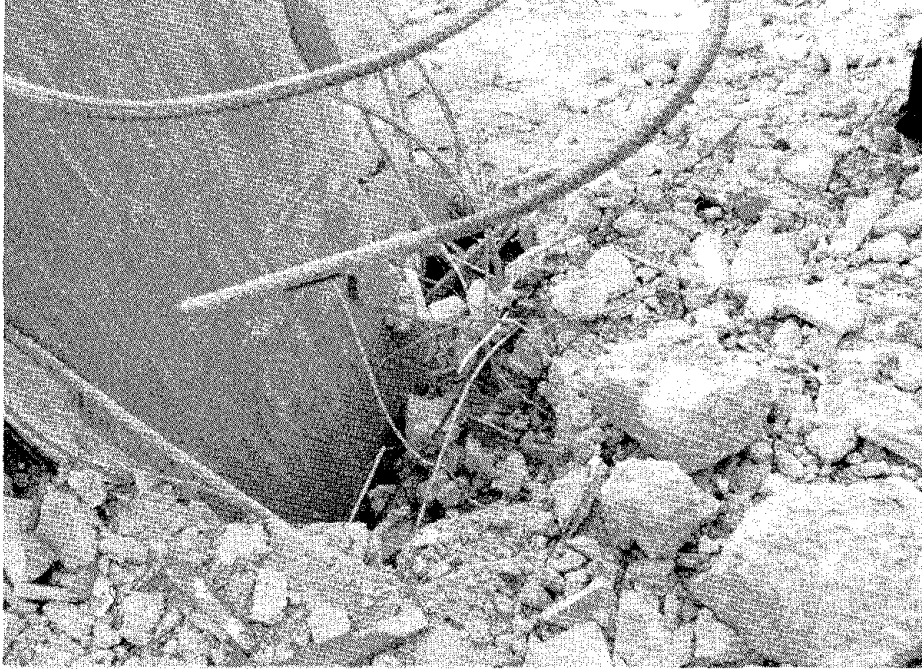
FIGURE 6.33 Apollo Hotel in Loutraki. The slabs sheared away from the column walls and came down one on top of the other.
