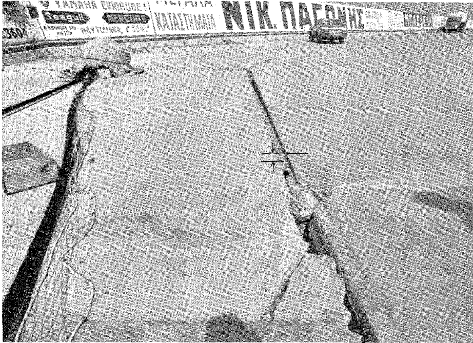
FIGURE 5.25 Jetty in Kiato. The expansion joints between the concrete blocks have been damaged. Note the differential settlement of about 20 to 30 cm.
