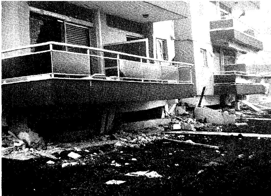
FIGURE 5.3 Failure of first-story columns.
