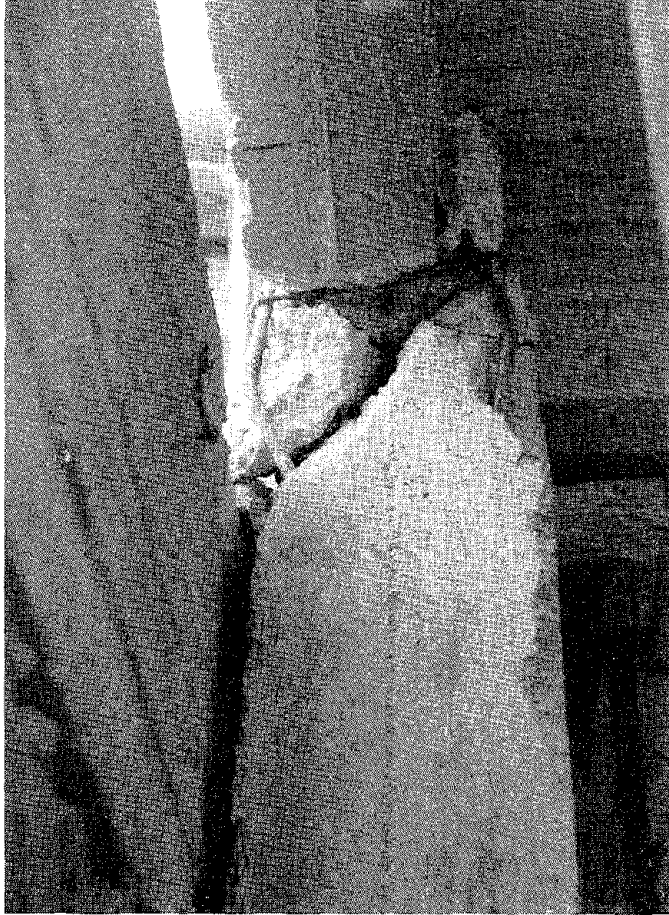
FIGURE 4.21 Detail of the damaged column in Figure 4.20. Note the gap between the two buildings after the earthquake.
