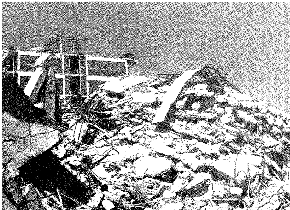
FIGURE 5.26 Collapse of nearly completed hotel in Vrahati.
