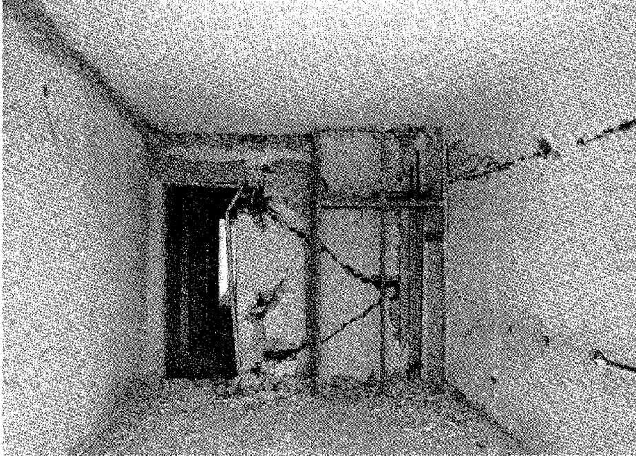
FIGURE 6.24 Galaxy Hotel in Vrahati. Inside view of a room in the second story of section III. The front brick wall extends along the long axis of section III (northwest to southeast).
