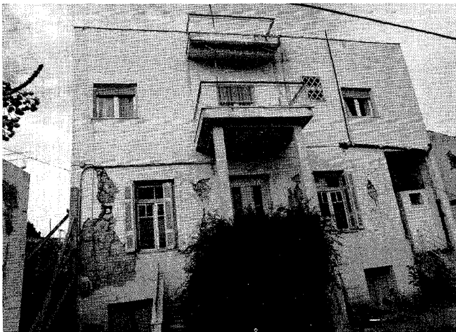
FIGURE 4.4 Additions are very vulnerable, as in this case in Megara. Usually the old building (the lower one) suffers most of the damage.
