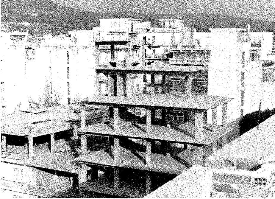
FIGURE 4.15 Eccentrically located walls in reinforced concrete frame under construction. This is a typical example of a drastic change in the plan area in a penthouse. Collapses of such penthouses were reported.
