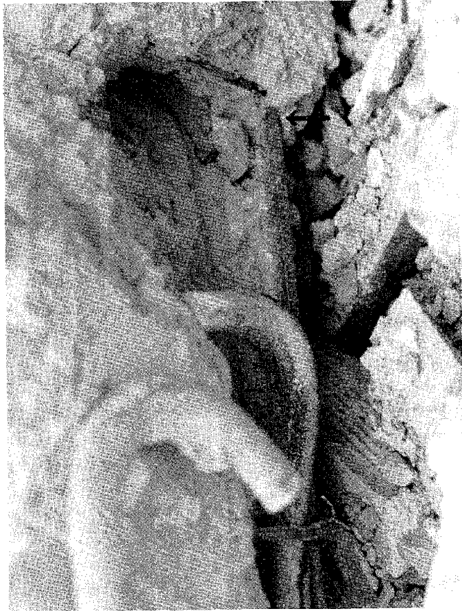
FIGURE 5.35 Detail of the collapsed hotel in Kineta. Note the slip of the hook and necking of the longitudinal bar (arrow).
