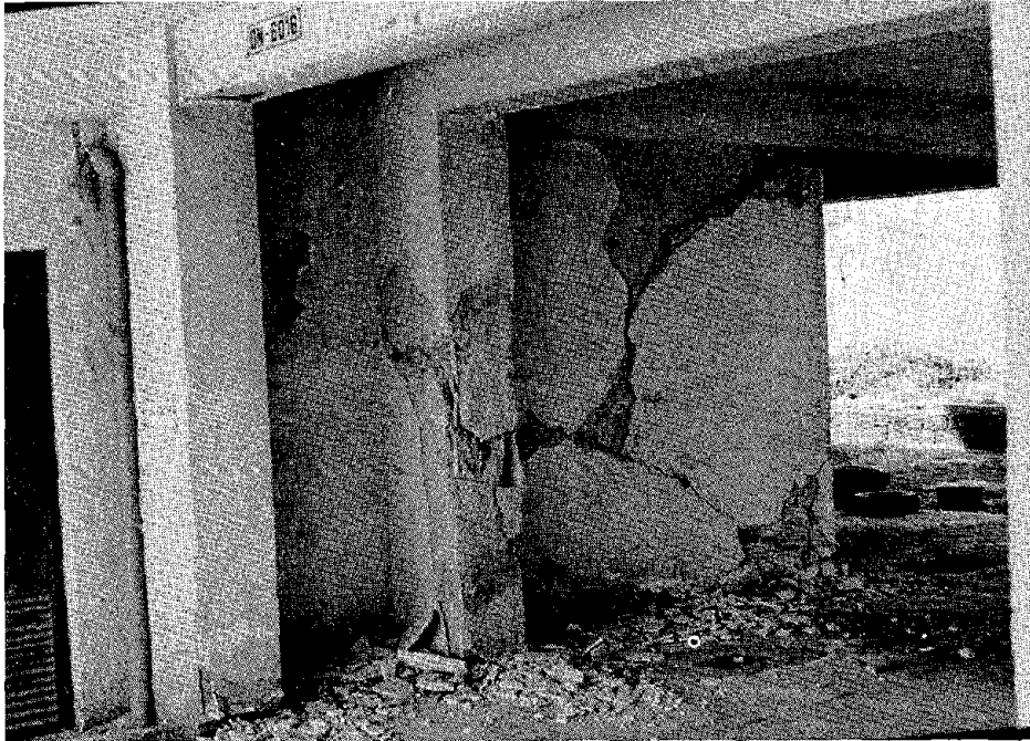
FIGURE 4.30 Typical shear failure of reinforced concrete column confined by a brick wall. The rupture of the masonry extends through the column.
