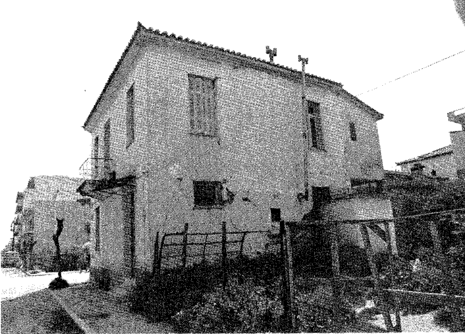
FIGURE 5.29 Many earthen buildings are about 100 years old. They have experienced two to three earthquakes as strong as the present ones and only needed the plaster surface repaired (although the repairs were not always done).
