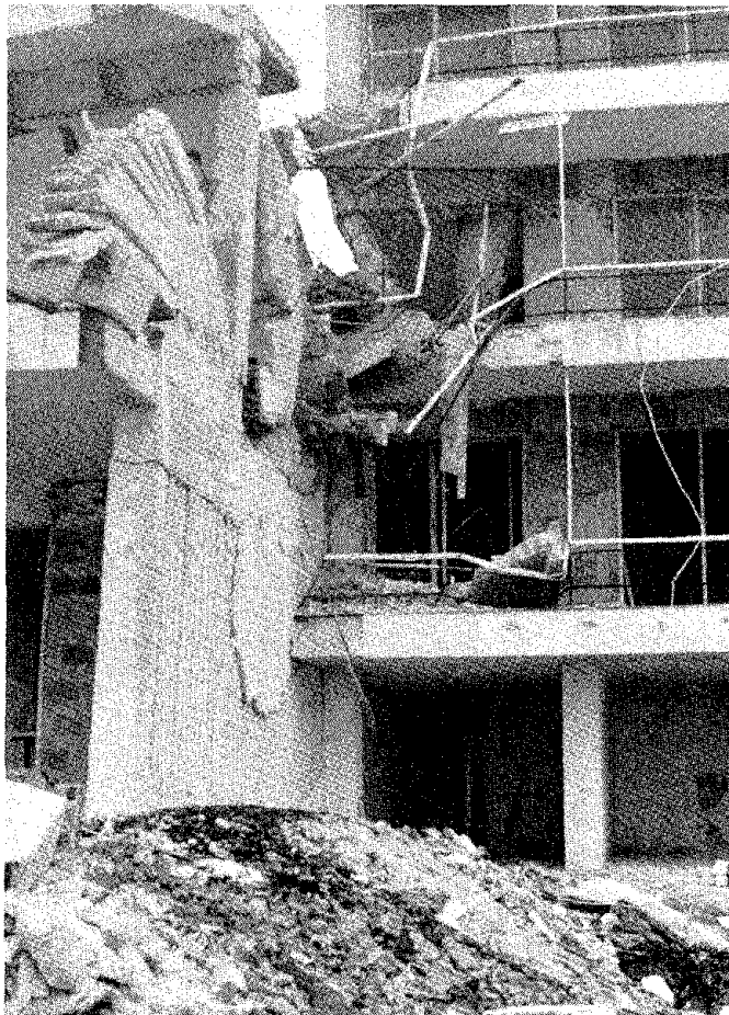
FIGURE 6.21 Galaxy Hotel in Vrahati. North side of the expansion joint between sections II and III.
