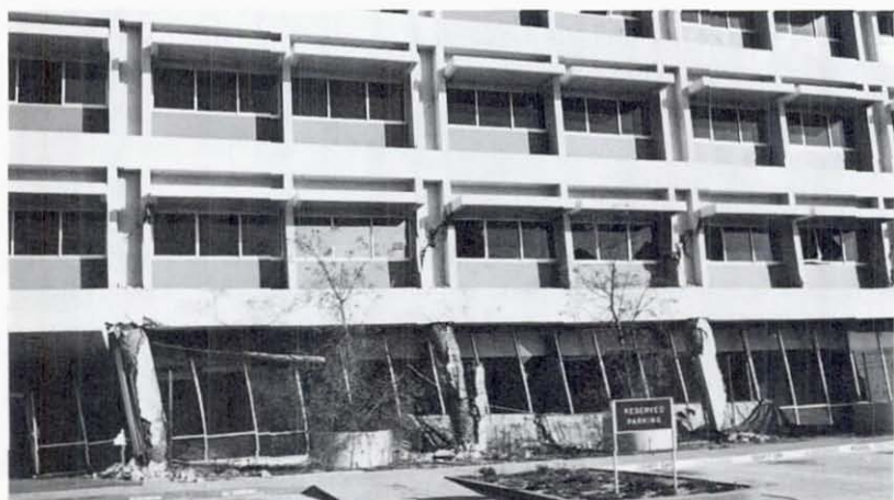
The new Olive View Hospital building was overstressed by the San Fernando earthquake. The damage was so severe that the structure was later demolished. The building had been designed according to the 1968 building code, but clearly the design was not adequate for the strong shaking it experienced.
