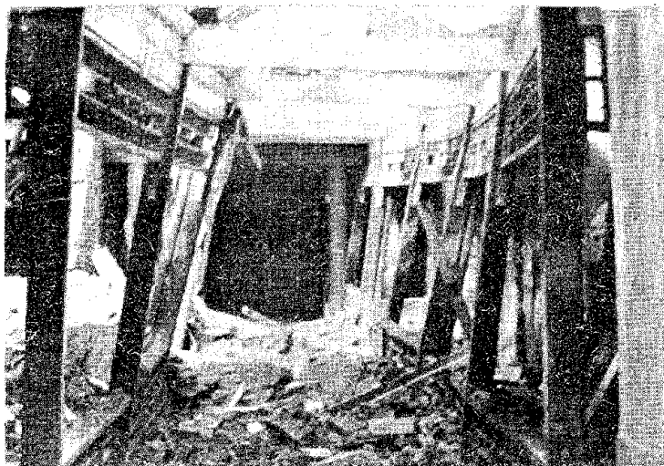
Fig. 10. Destructive building seriously, Tianjin-Hotel.
