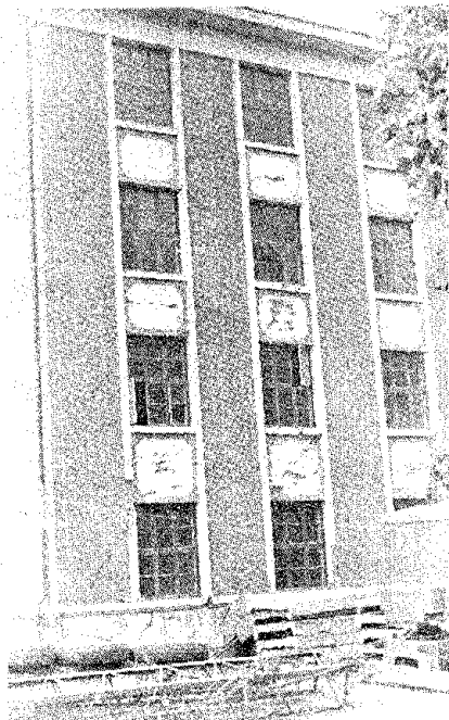
Fig. 6 Damage to building Having sunk spandrel wall during the Tangshan earthquake
