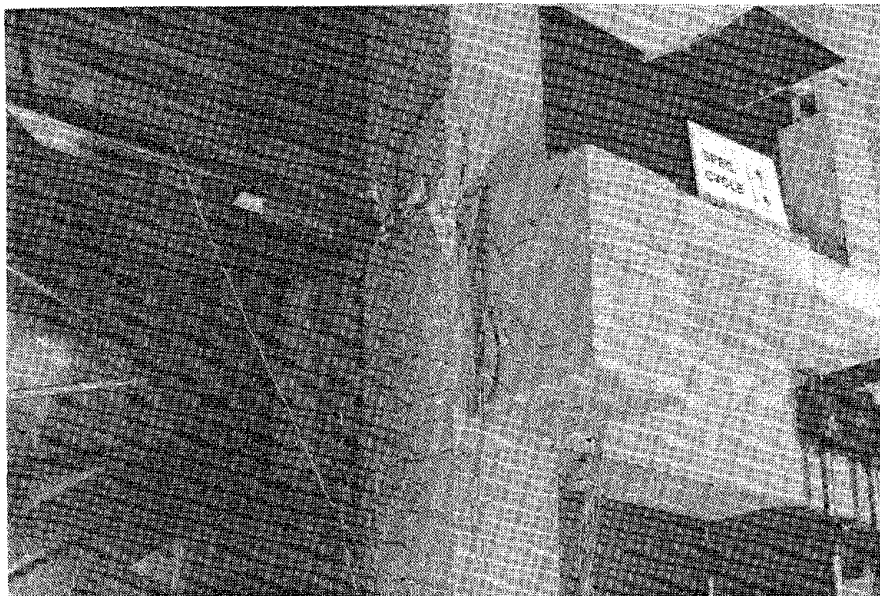
Fig. 3.29. Crushing of the Concrete Due to the Hinging of the Upper Column Half - Specimen 6.
