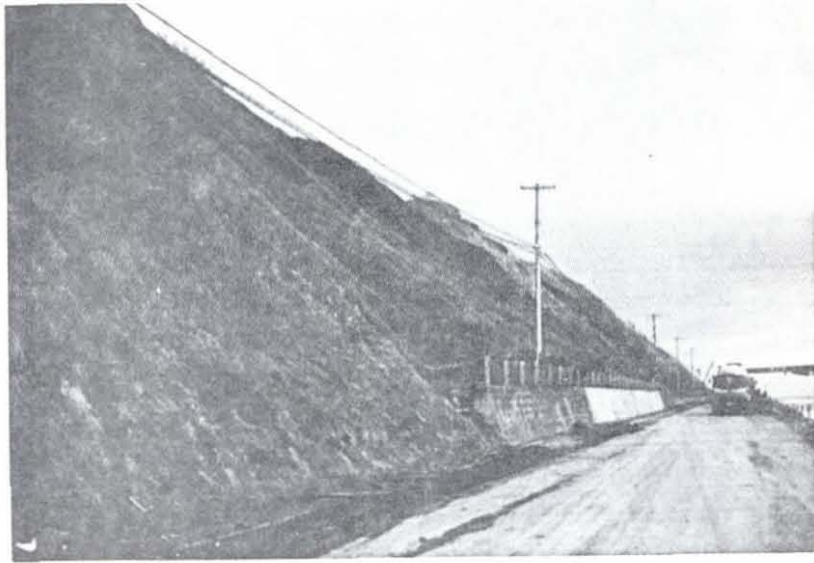
Photo. 3 Light Damage to Slope along National Highway Route 235, at Irifune Area, Shizunai Town. Retaining Walls Protected from a Large Failure.
