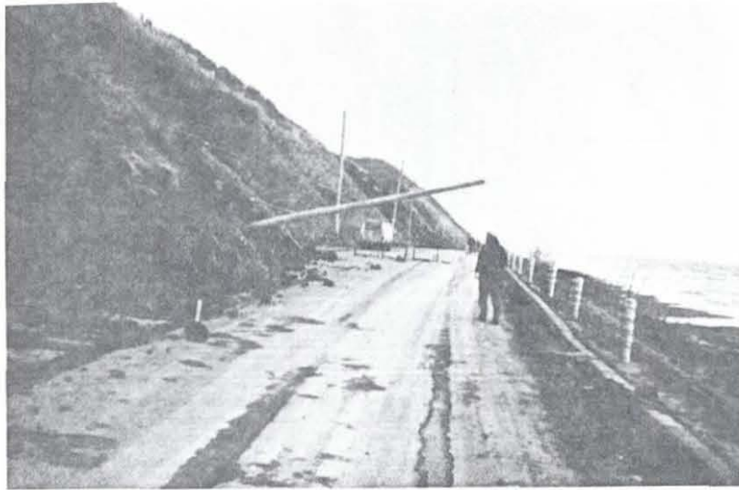
Photo. 1 Damage to Slope along National Highway Route 235, at Irifune Area, Shizunai Town. An electric post was overturned.
