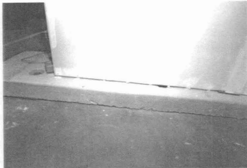
Figure 6: Specimen PD3-V Run No. 1 Test No. A-3, Frequency = 0.5 Hz Peak Command Displacement = \pm 3/8 Inch Typical Damage @ Bottom Edge Nailing Crumbling of Gypboard Around Nail Heads
