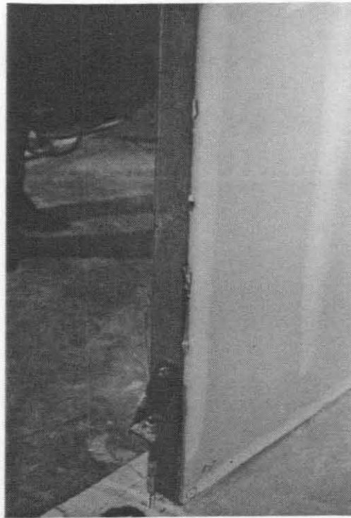
Figure 41: Specimen PD-4 Run No. 2 Popping of Nail-Heads in Gypboard @ End Studs Test No. A-8, Frequency = 0.5 Hz Peak Command Displacement = \pm 1\frac{1}{2} Inches
