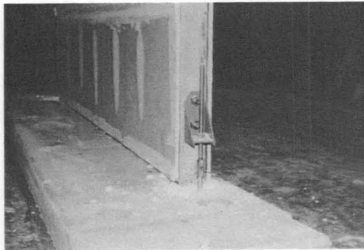
Figure 24: Specimen PD3-H Damage @ Left Holddown and @ Sill-Plate - Separation Between Gypboard and End Studs and Crumbling of Gypboard Around Nail Heads @ Sill-Plate
