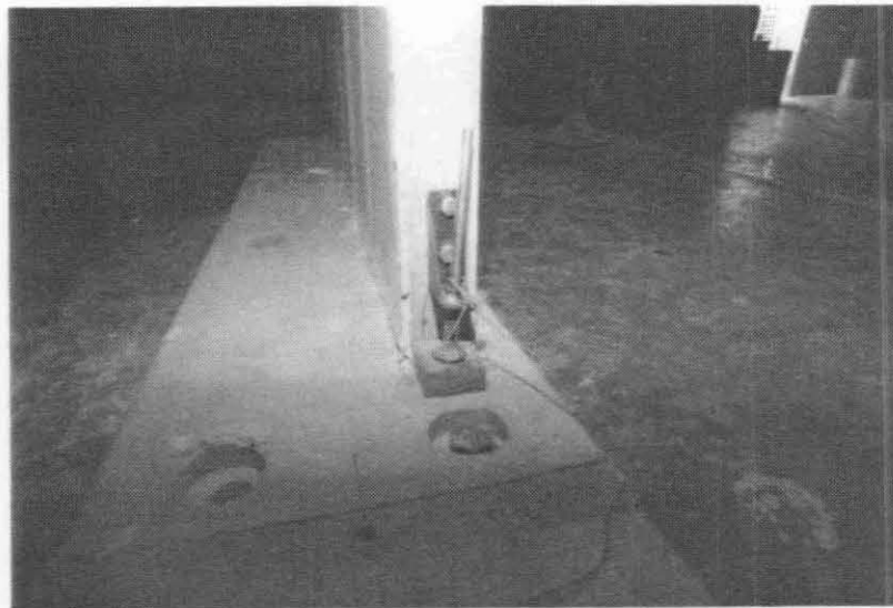
Figure 10: Specimen PD3-V Run No. 2 Simpson HD-5 Holddown @ South End Typical Damage Consists of Crumbling of Gypboard @ End Studs Through Working of Nails
