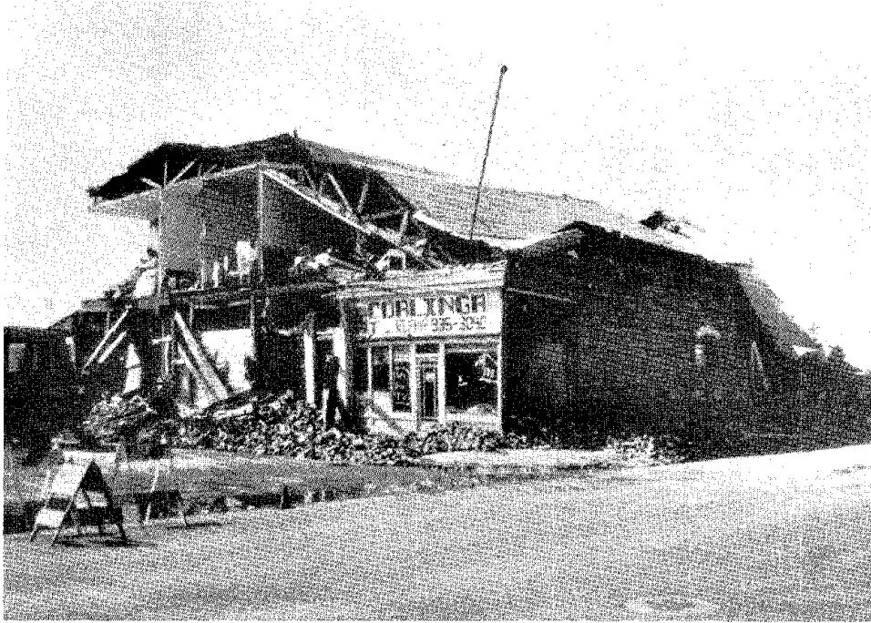
FIGURE 12 Structural damage in the Coalinga business district resulting from the May 2, 1983 earthquake (M6.5). Source: California Division of Mines and Geology (1983). (Photograph by James Stratta)
