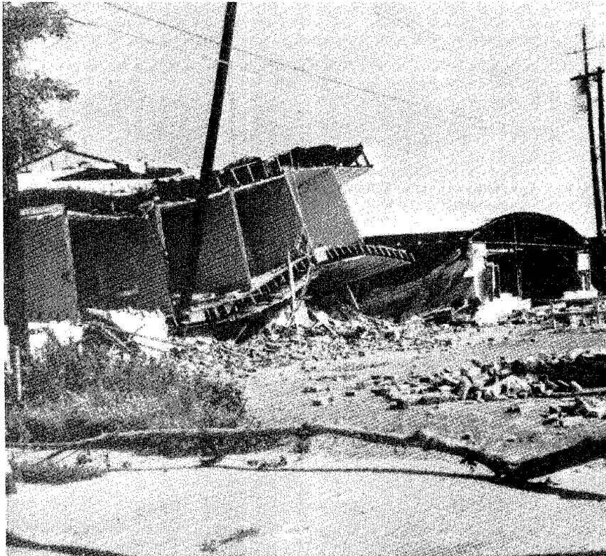
FIGURE 13 Structural damage to a brick building resulting from the Coalinga earthquake of May 2, 1983. The epicenter of this magnitude 6.5 shock was about 10 miles from the town. Such buildings, not designed to resist earthquakes, are very vulnerable to damage. Source: California Division of Mines and Geology (1983). (Photograph by James Stratta)
