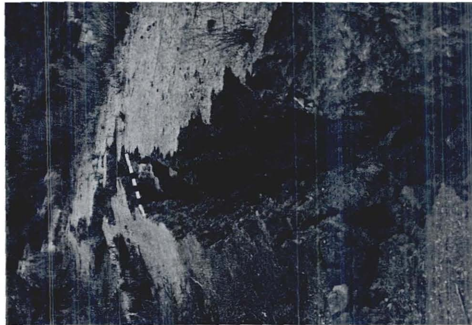
(a) Cracking in Slope of Dam
