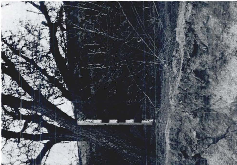
(b) Slumping of Crest of Dam--tree was formerly on crest of embankment
