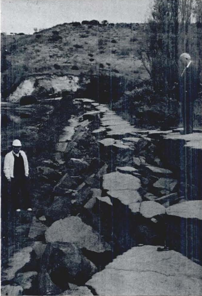
Fig. 2 CRACKING AND SLUMPING IN UPSTREAM SLOPE OF LA MARQUESA DAM
