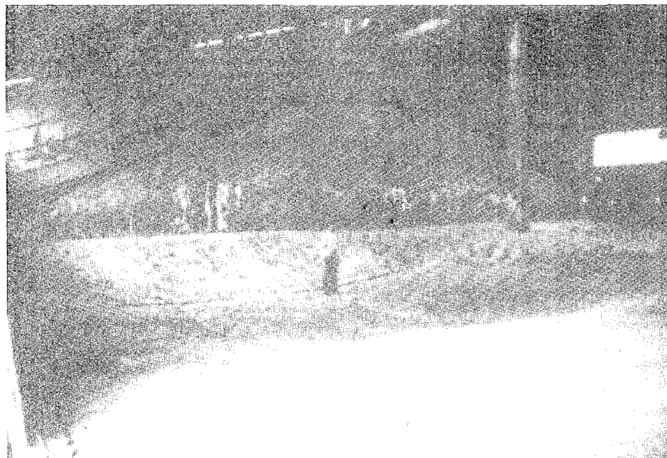
Figure 3.4 - Slab on Grade Settlement Due to Liquefaction (Bertero, et. al., 1985)
