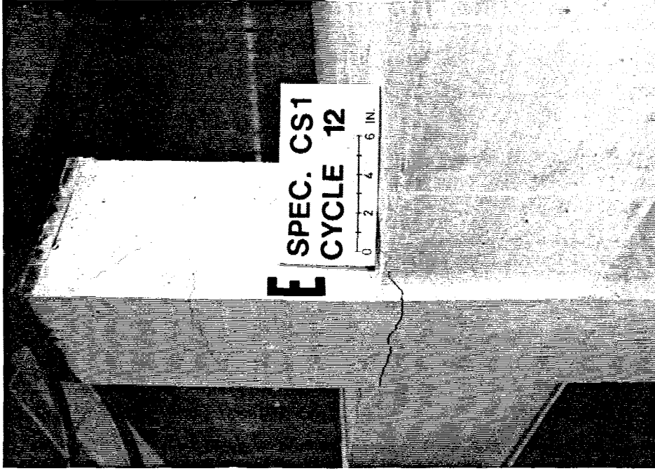
Fig. 3.10(b) Flexural Cracks in Exterior Column of Specimen CS1
