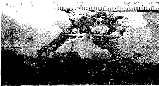
Photo. 4 Damage of the Pile of S-building
