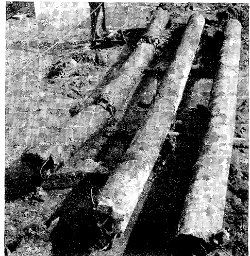
Photo. 3 Deformed Shapes of the Piles of S-building
