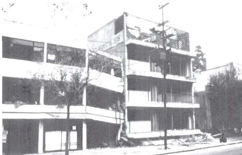
Figure 7. Foundation failure: right hand building settled almost a full story height pulling down adjoining part of left hand structure.
