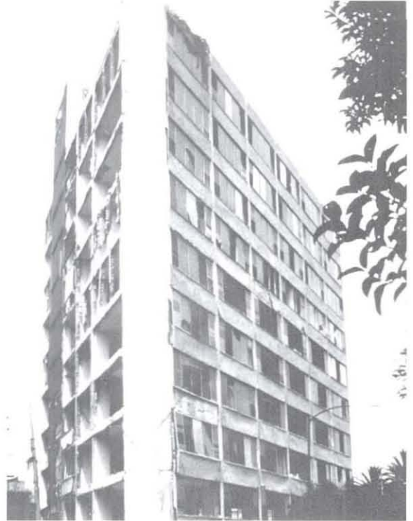
Figure 9. Lower story failure of corner building having triangular footprint.
