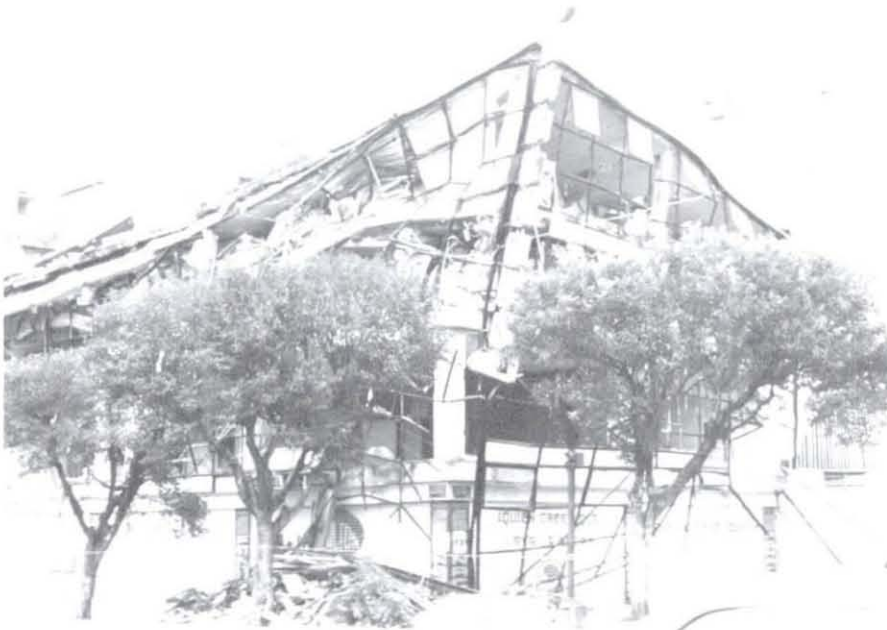
Figure 10. Failure of corner building indicating torsional motion.
