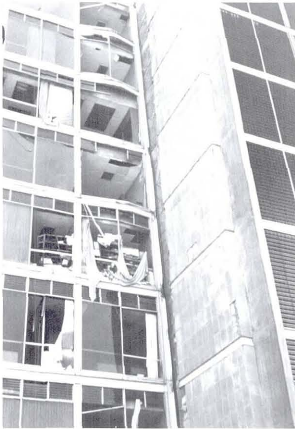
Figure 5. Evidence of pounding: steel beams in upper level permanently bucked outwards.
