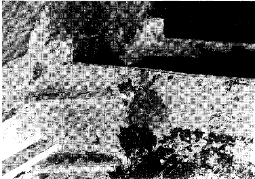
(c) East Flange of Link Near Column- After Testing (Note cracks in flange at ends of ribs)
