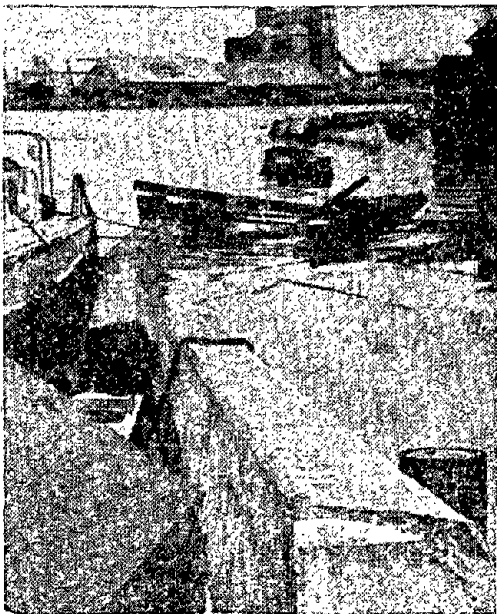
Photo 19 Damage to the Quay Wall on the Right Bank of the Old Kurinoki River (Point ② in Figure 22(a))12)
