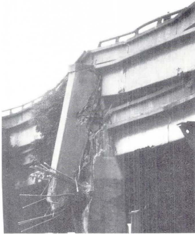
Fig. 1.14 Close-up view of failed column.
