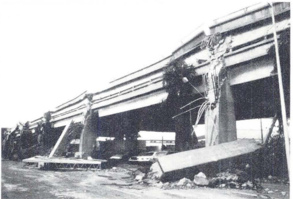
Fig. 1.13 Collapse of the I-880 Cypress St. Viaduct, illustrating the 'popping out' of the second story columns.
