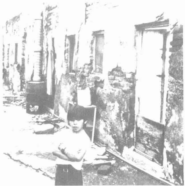
Figure 3.5.4. Deteriorated and earthquake damaged housing in central Mexico City.
