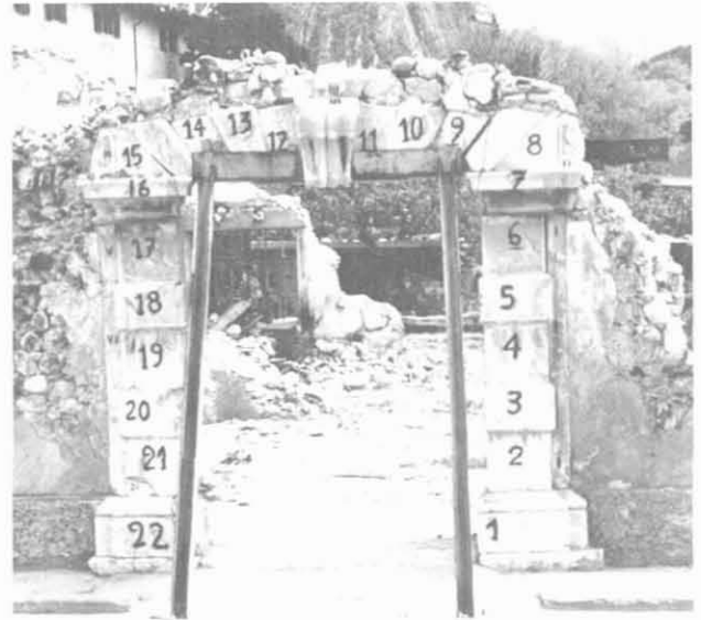
Figure 3.3.8. Arch stones of a Gemona villa numbered for accurate replacement when the gate is rebuilt. Photo, taken in 1978, is courtesy of the Earthquake Engineering Research Institute.
