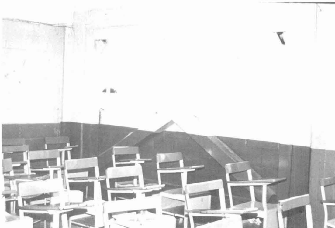
Figure 3.5.11. School classroom reinforced with X-bracing.
