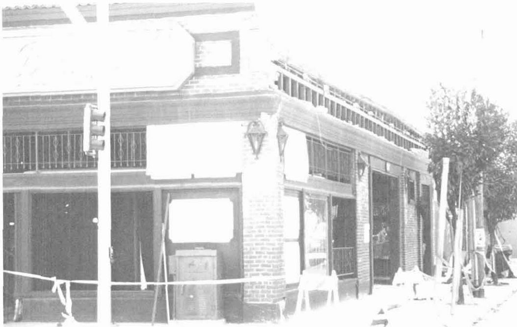
Figure 4.3.12. Downtown buildings damaged in earthquake.
