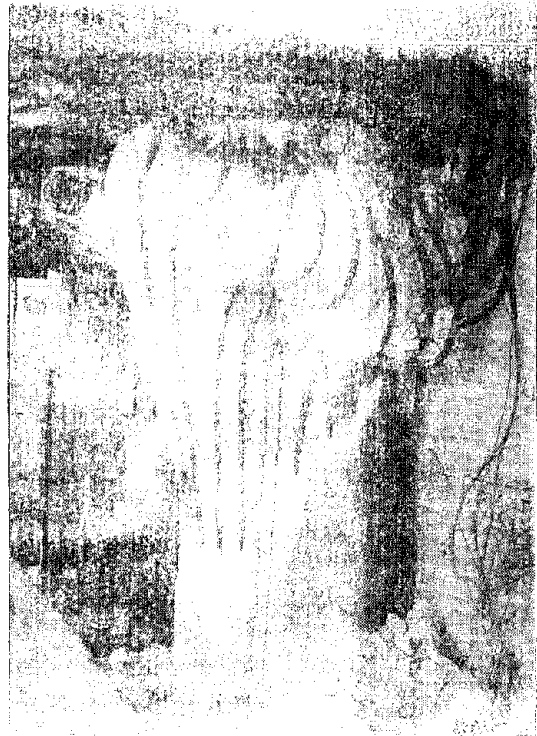
Photo 4.8 Damage of Columns of Genega/Channel Bridge
