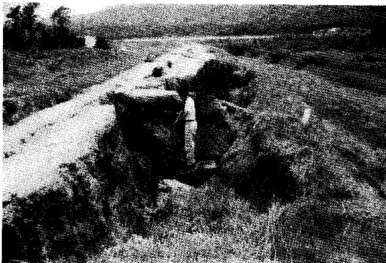
Photo 6.1 Damage to Hatsuta Dike (Shiribetsu River, Right-Side Dike)
