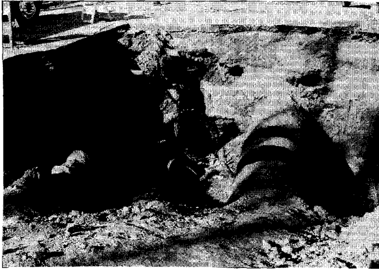
Photo 7.6 Rupture of Gas and Water Pipes due to Tension (Balboa Street, Granada Hill)
