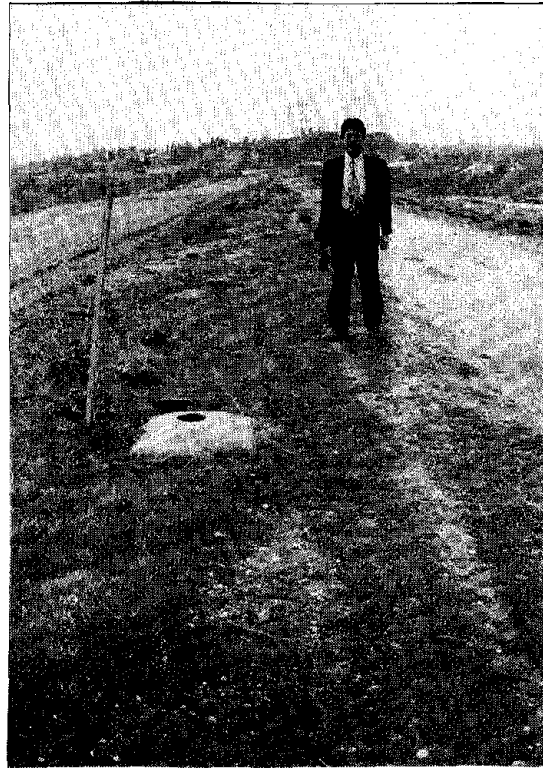
Photo 7.4 Cracks on Crest of Lower San Fernando Dam (Aqueducts Plant, DWP, City of Los Angeles)
