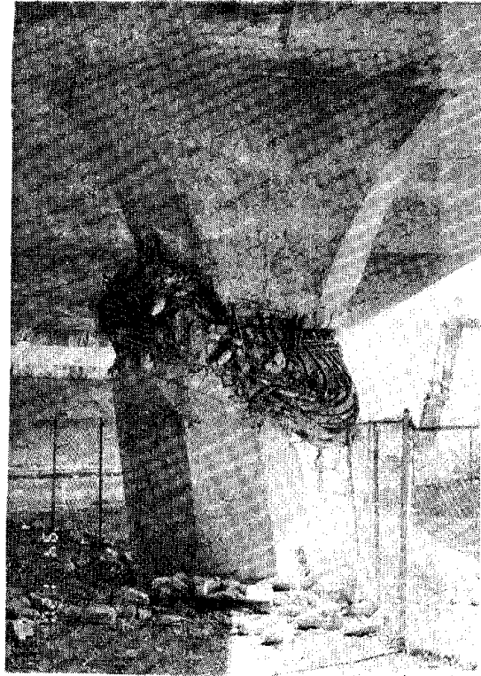
Photo 4.5 Dislodgement of Column Axis due to Shear Failure (S-118 Mission/Gothic Undercrossing)
