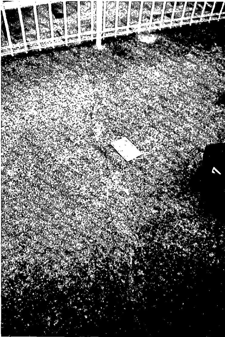
Figure 5.15: Old crack observed on crest of Karasuhara Dam.
