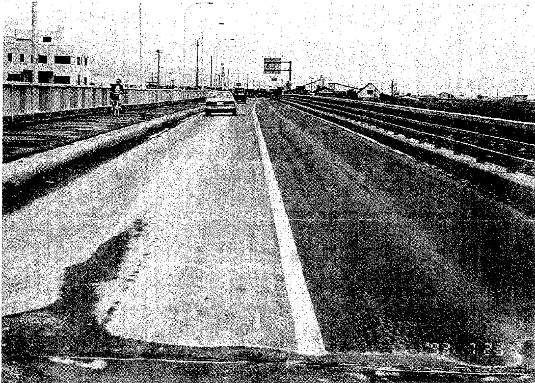
Photo 17 Residual Displacement found at the Deck caused by the Inclination of Piers (Osyamanbe Bridge)
