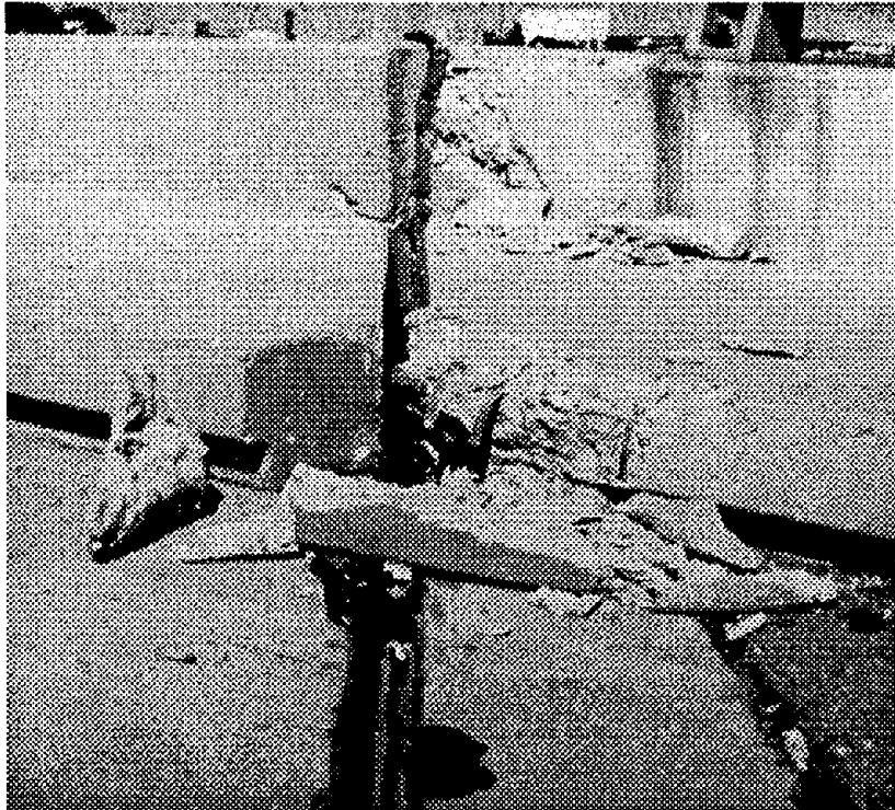
Figure 20. Damage at Whitewater O.C. Abutment 1 Expansion Joint
