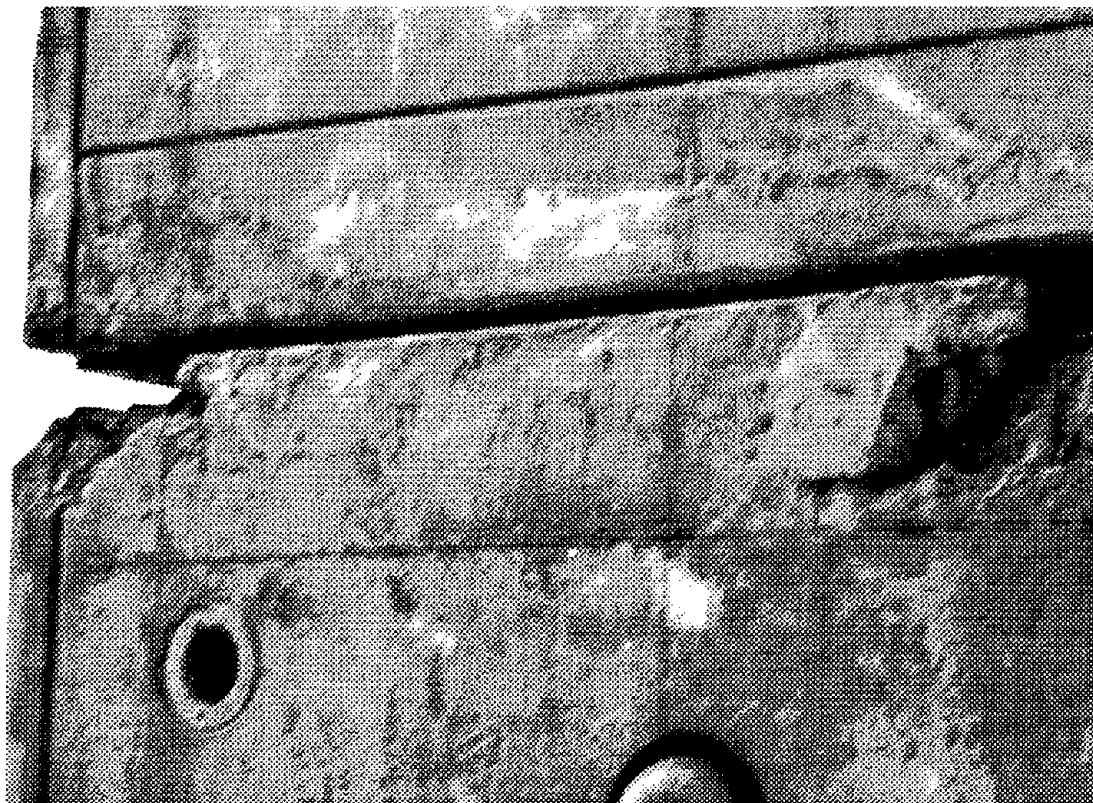
Figure 39. Looking up at Bridge Soffit Damage from Hinge Diaphragm Punching Shear Failure
