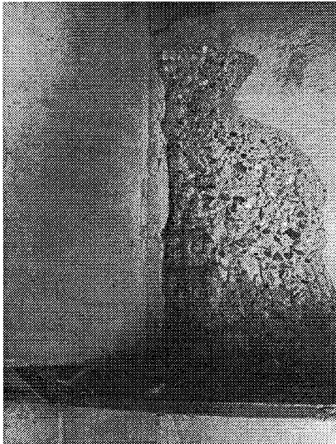
Figure 32. Napa River Bridge Earthquake Damage at Fixed Joint
