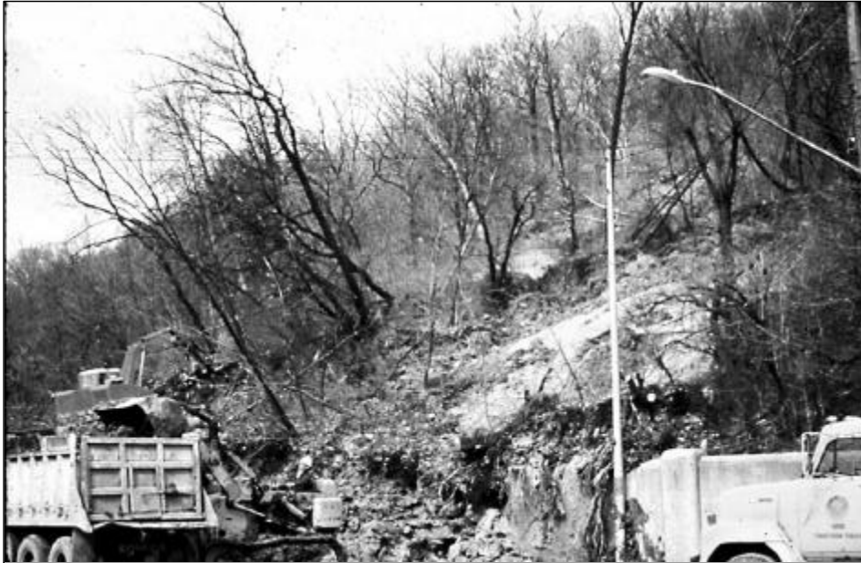
Earthflow in Cincinnati, Ohio. Material being removed by highway crew.
