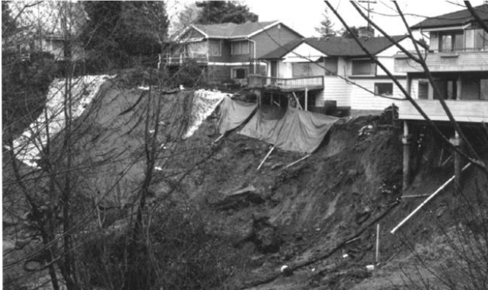
Landslide in northwest Seattle, Washington. Foundation of house on right edge of photograph and decks of neighboring houses have been undermined. (Photo by Alan F. Chleborad, USGS)
