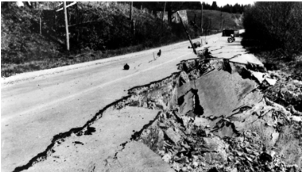
Figure 207. Damage to Black Lake Road south of Olympia, Wash. (pl. 5, loc. 44), caused by failure of a steep lake bank during the earthquake of April 13, 1949. Photograph used by permission of Jack Goldsby, Tumwater, Wash.
