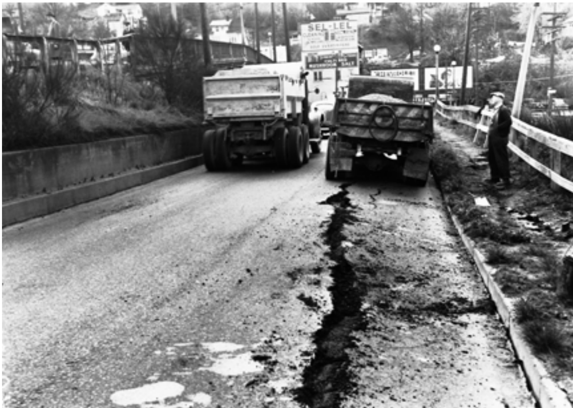
Figure 193. Ground failure along Spokane Street approach to West Seattle (pl. 4, loc. 16) triggered by the April 13, 1949, earthquake. Pavement cracks and slight slump are in a road embankment composed of artificial fill. Note arcuate scarp and tilted light pole at right. Photograph from the Seattle-Post Intelligencer Collection, courtesy of the Museum of History and Industry, Seattle, Wash.
