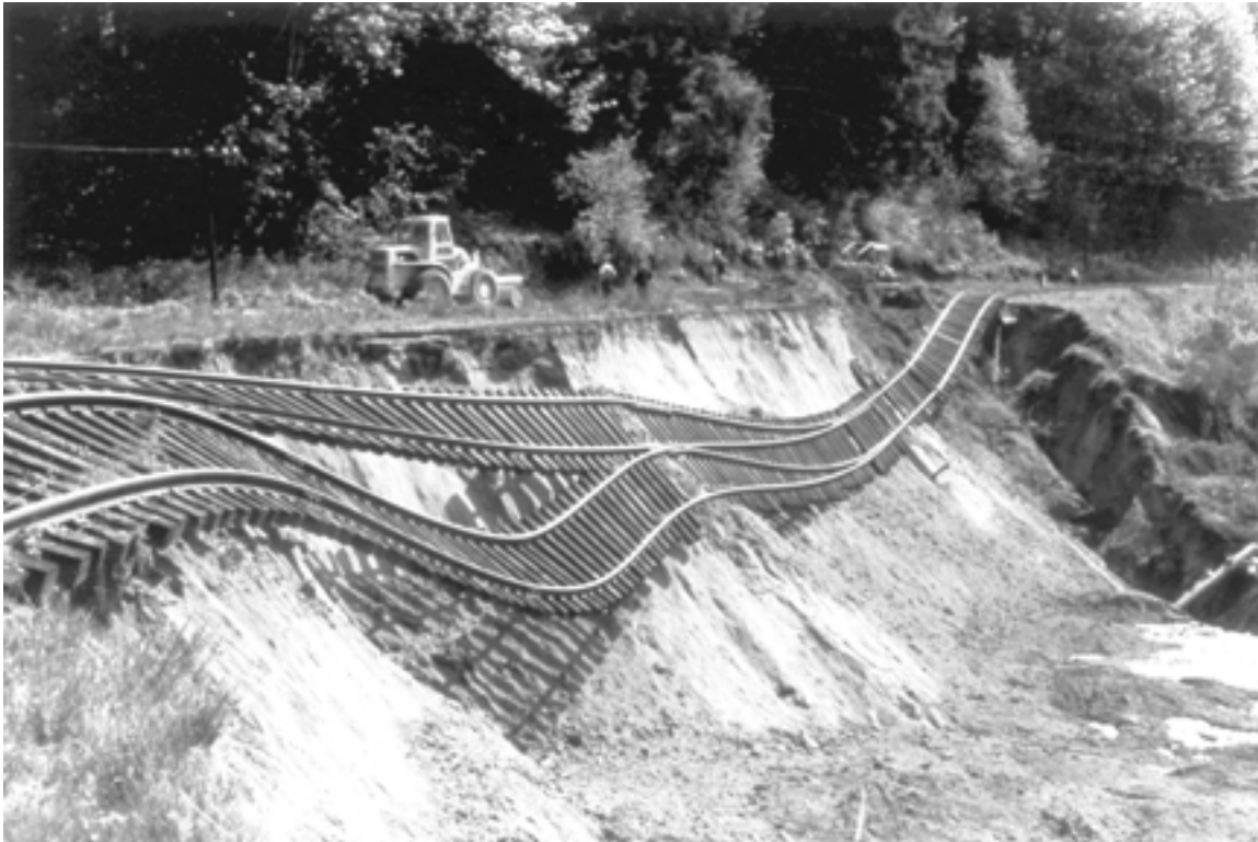
Figure 206. Damage to Union Pacific Railroad tracks near Tumwater, Wash. (pl. 5, loc. 45), due to a 1965 earthquake-induced slope failure in artificial fill. Photograph by Gerald W. Thorsen, Division of Geology and Earth Resources, Washington Department of Natural Resources, Olympia, Wash.
