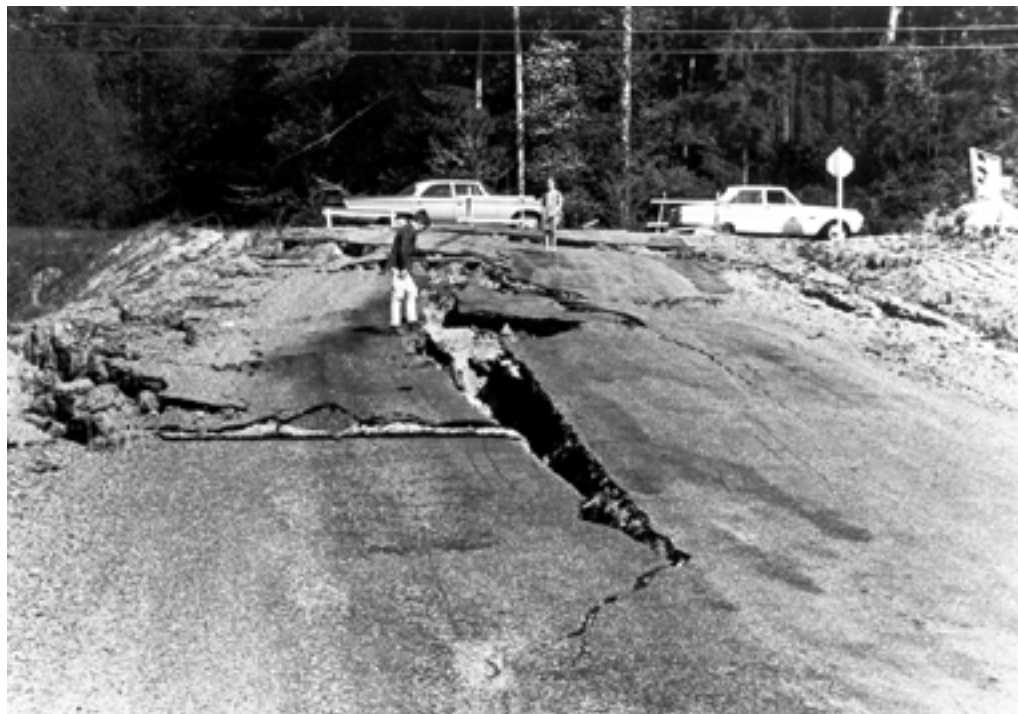
Figure 198. Damage to Country Club Road, southwest of Port Orchard, Wash. (pl. 4, loc. 2), due to slumping induced by the April 29, 1965, earthquake. This slump occurred in granular fill underlain by glacial deposits of the Vashon Drift. Photograph used by permission of the Bremerton Sun.
