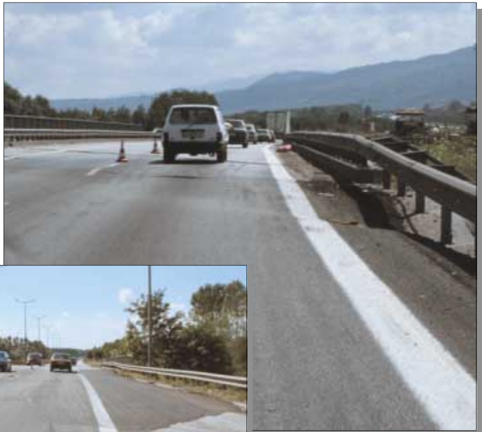
Figure 52. Densification of dry approach fill adjacent to bridges of the Trans European Motorway was widespread and caused disruption of the roadway. Immediately following the earthquake, Turkish highway engineers placed asphalt ramps on the roadway to reduce the hazard. Photographs by Thomas L. Holzer.
