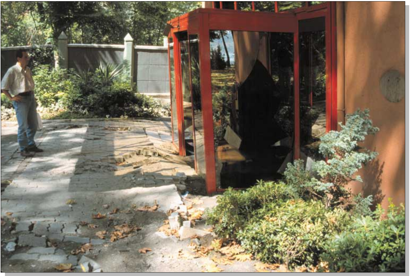
Figure 38. Sunken entryway into Sapanca Hotel created when building sank into liquefied soil. Photograph by Thomas L. Holzer.
