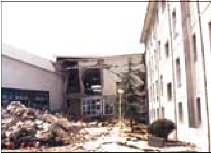
Figure 44. Damage to Officer's Club on Turkish Naval Base, Gölcük, which was located directly on the surface fault rupture. Photograph by National Institute of Standards and Technology.
