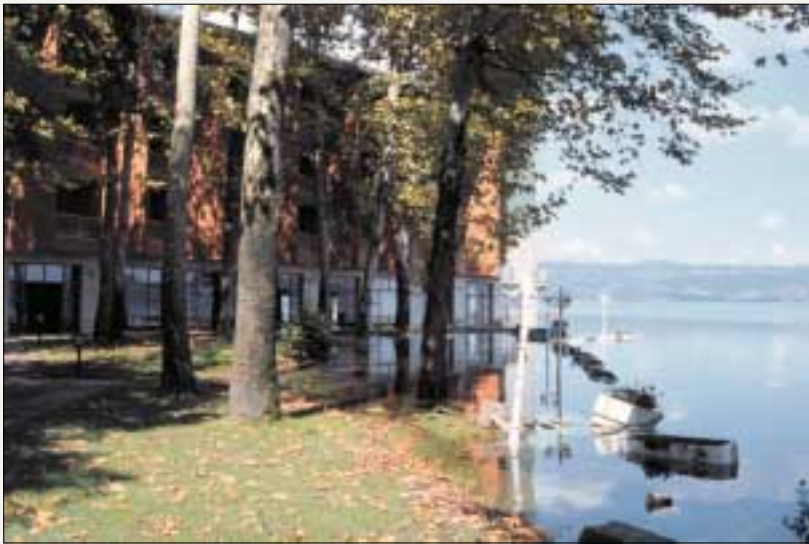
Figure 37. Submergence of shoreline at Lake Sapanca and settlement of Sapanca Hotel. "Moat" adjacent to wall indicates the hotel has sunk into the ground because of liquefaction of underlying sandy soil. Photographs by Thomas L. Holzer.
