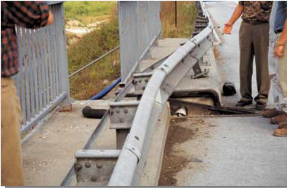
Figure 51. Ground shaking caused the westbound span of the Sakarya River bridge to displace 50 cm relative to the east abutment. This was the largest permanent displacement caused by shaking at any bridge. Photograph by Selcuk Toprak.
