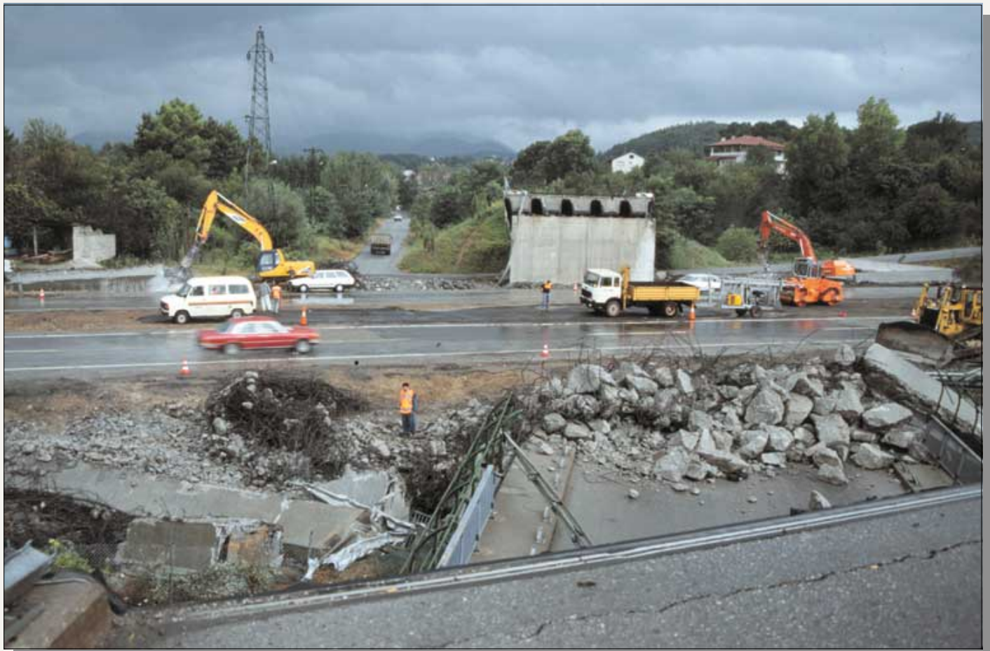
Figure 53. The Arifiye overpass collapsed because the surface fault rupture passed directly through its north abutment (foreground). Ten riders of a bus were killed when the bus collided with the collapsed overpass. Photograph by Thomas L. Holzer.
