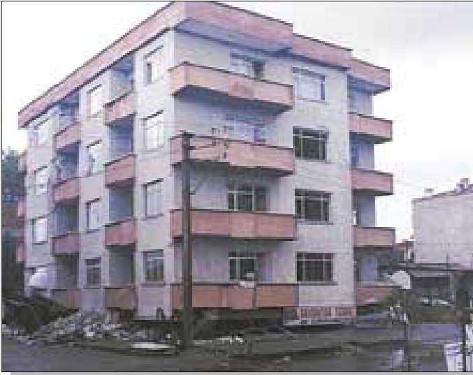
Figure 41. Partial building collapse in Yalova as the result of shear failure of first story columns. Photograph by National Institute of Standards and Technology.
