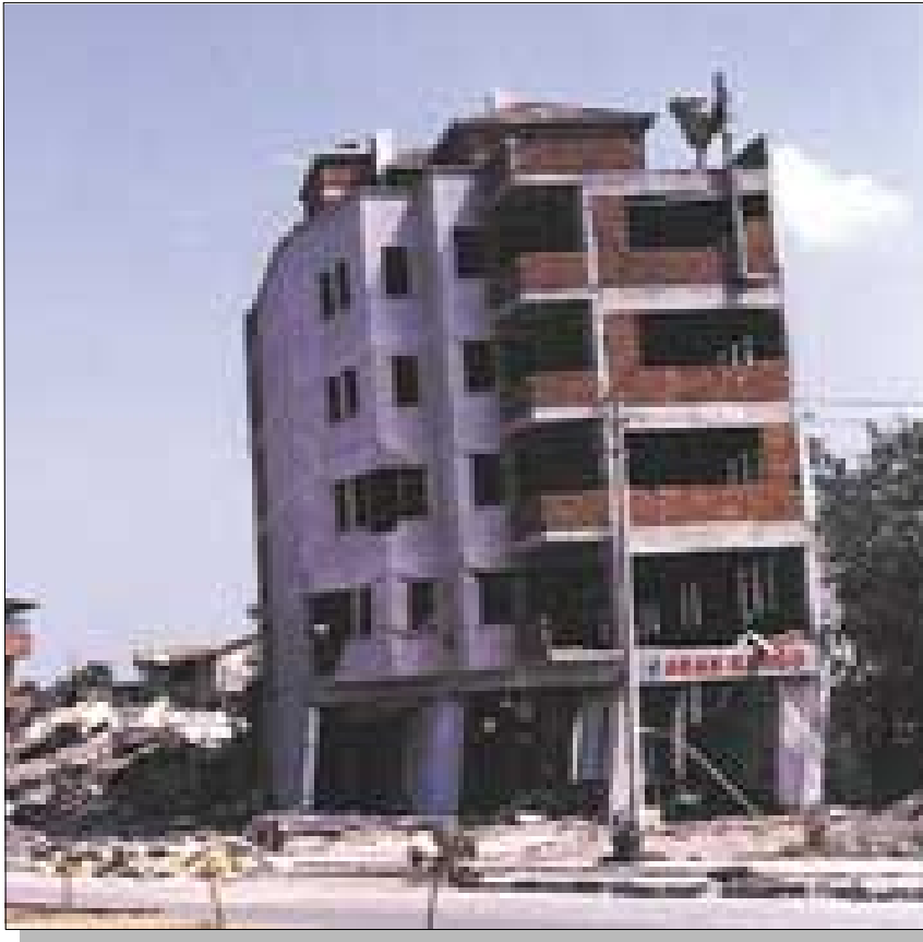
Figure 43. Near collapse of building in Adapazari as the result of formation of column hinges in the first story. Photograph by National Institute of Standards and Technology.
