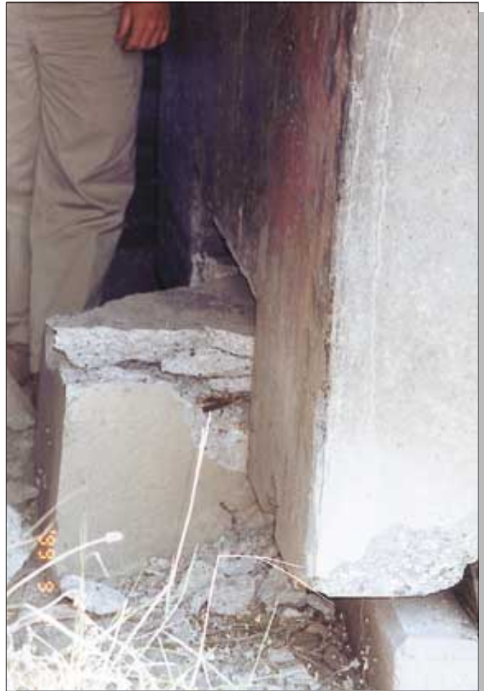
Figure 50. Failure of shear keys was common at bridges of the Trans European Motorway. Shear keys at the end of girders prevent transverse and longitudinal seismic movements. Photograph by Selcuk Toprak.
