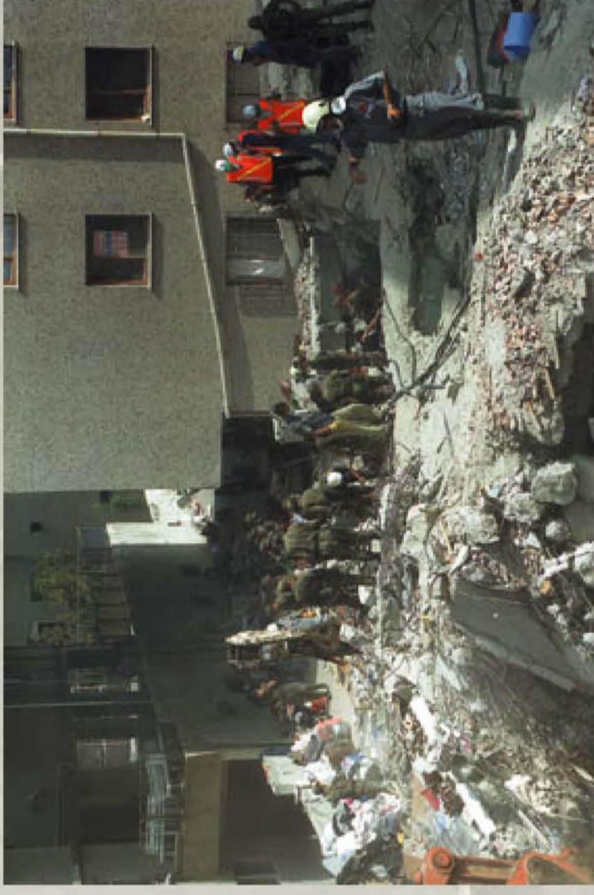
Figure 31. Rescue effort 4 days after the main shock at a collapsed building in area of concentrated damage in Avcilar. Photograph by Thomas L. Holzer.
