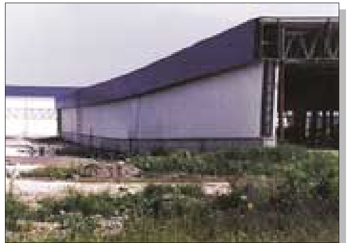
Figure 45. Industrial building damaged by near-fault ground movements east of Gölcük. Building is on downthrown block of normal fault and near a major change of strike in the surface fault scarp. Photograph by National Institute of Standards and Technology.
