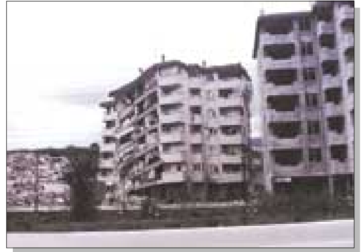
Figure 42. Partial collapse of building near Izmit as the result of shear failure of intermediate columns. Note various stages of damage despite apparently similar construction. Photograph by National Institute of Standards and Technology.
