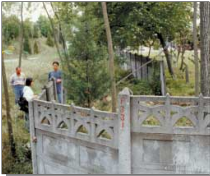
Figure 18. Offset wall near Arifiye. The right-lateral displacement is 4.58 m. Photograph by Heidi Stenner.
