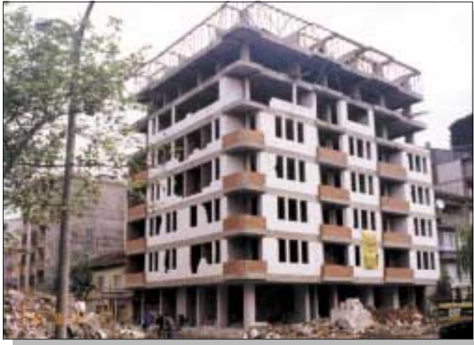
Figure 40. Building in Izmit under construction using reinforced concrete frame construction. Note absence of shear walls. Photograph by National Institute of Standards and Technology.
