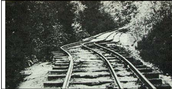
Figure 3-7. Damage to the railroad track between Wrights Station (near the tunnel) and Alma caused by the 1906 earthquake. Both historic settlements and the rail line no longer exist. The gravel road now follows the rail path. The photograph is from the Lawson Report.
