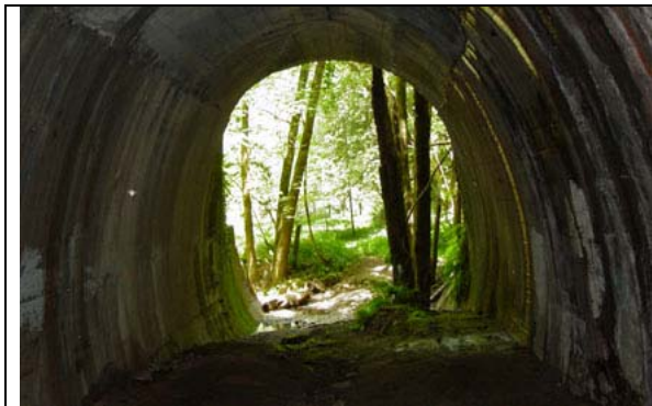
Figure 3-6. View looking out of the west end of Wrights Tunnel toward Los Gatos Creek. The tunnel is now full of leaking cracks that are feeding a small stream flowing from the mouth of the passage.
