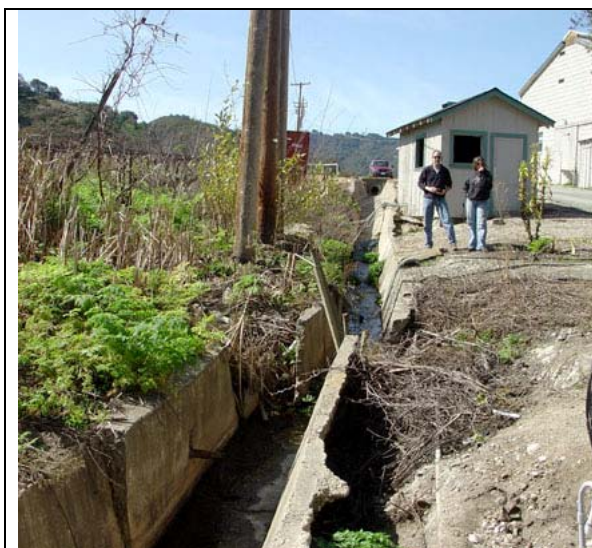
Figure 2-7. This cement-lined drainage ditch on the south side of the DeRose Vineyards shows offset from creep along the San Andreas Fault. The drain was probably constructed before the 1906 earthquake.
