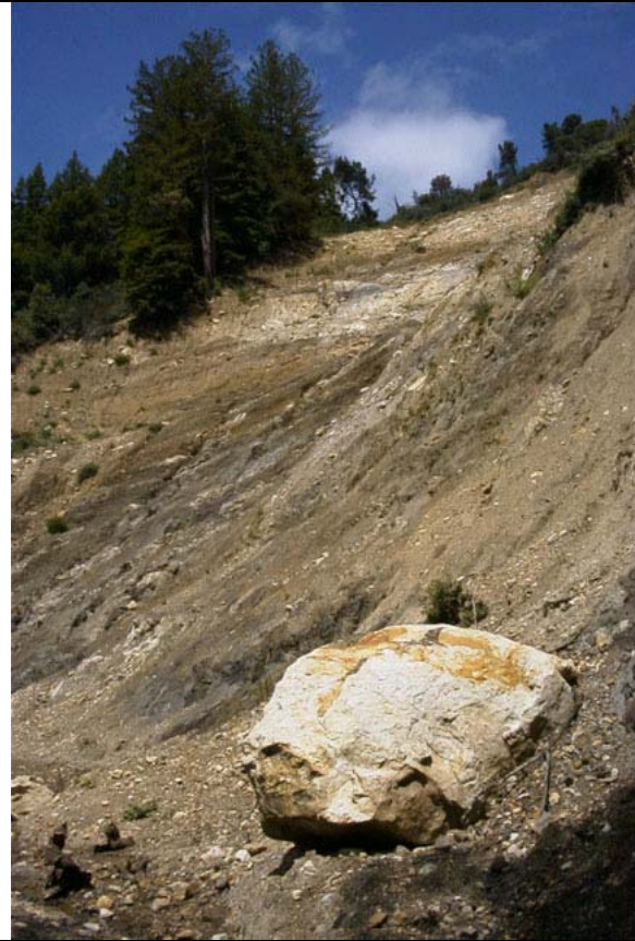
Figure 3-18. The Highland Way slide. Extensive work was conducted to remove dead trees and loose rock before the road could be repaired. This looser material is derived from Tertiary rock which consists of dark, hard, siliceous marine shale with interbedded arkosic sandstone. This sequence of marine strata forms a belt along the eastern side of the San Andreas Rift Valley for many miles extending to the south.
