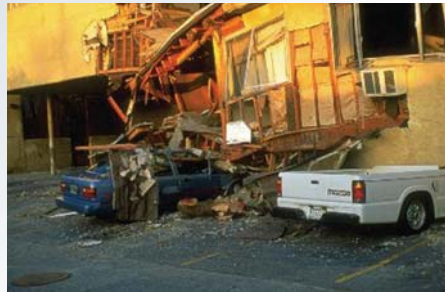
The “soft” first story of this apartment building collapsed in the 1994 magnitude 6.7 Northridge earthquake, crushing cars below and severely damaging the floors above (FEMA photo).
