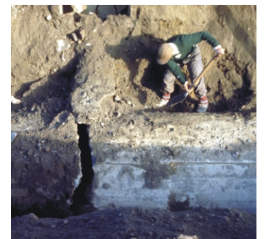
Broken sewer main, Puerto Montt.
