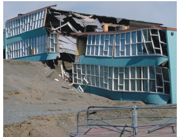
School torn by landslide, Anchorage.
