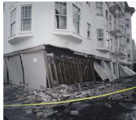
“Soft story” buildings, typically with parking on the ground floor, like the one pictured here, are common throughout the Bay Area and are particularly at risk when exposed to strong shaking (USGS photo).
