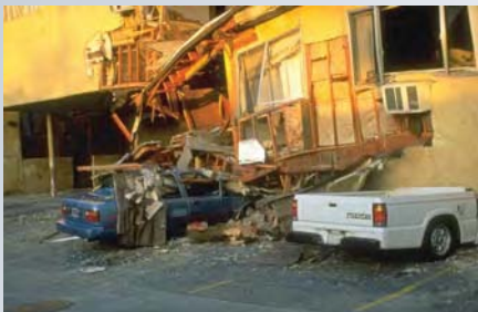
The first story of this apartment building collapsed, crushing cars below (FEMA photo).
