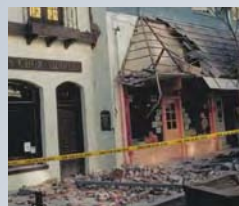
Businesses and rental properties may suffer serious damage (USGS photo).
