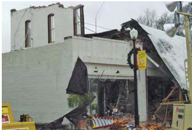
Collapsed roof in downtown Paso Robles following the San Simeon earthquake of December 22, 2003. Two people were killed by falling debris when they ran out of the building. (USGS photo)
